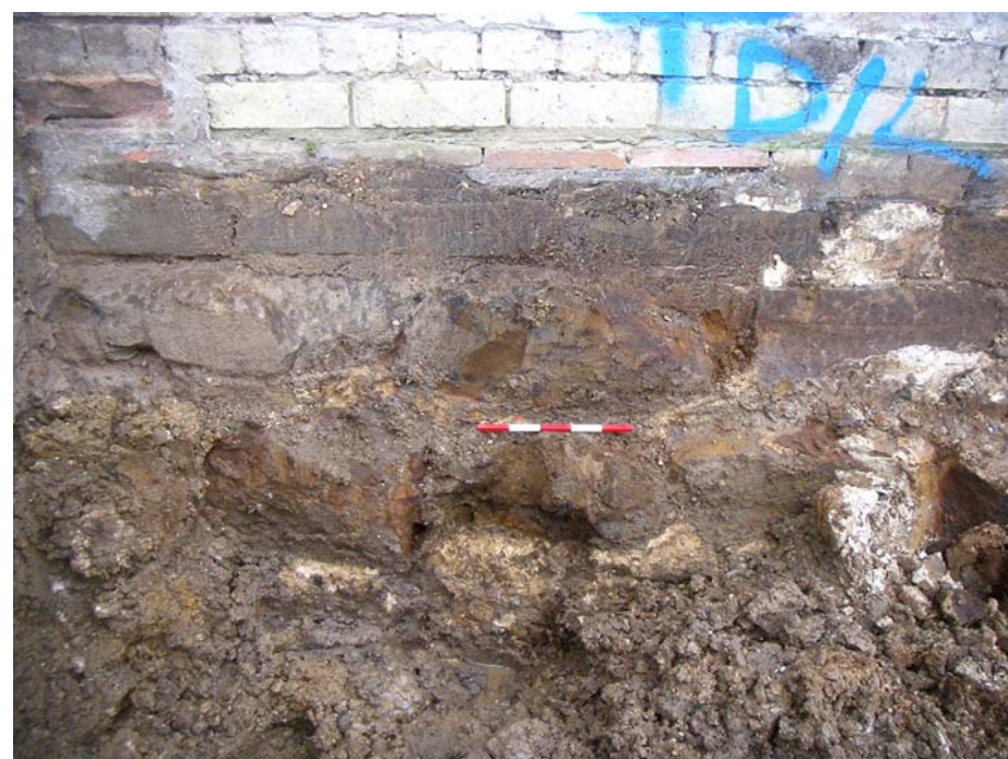
Image 10: Detail of the Ironstone footing seen in the top left corner of image 8. Scale 25cm in 5cm divisions.
