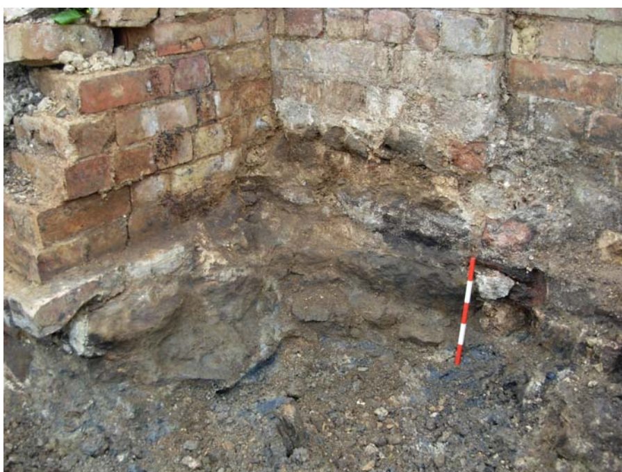
Image 12: Detail of the Ironstone footings of the ancillary building. Scale 25cm in 5cm divisions.
