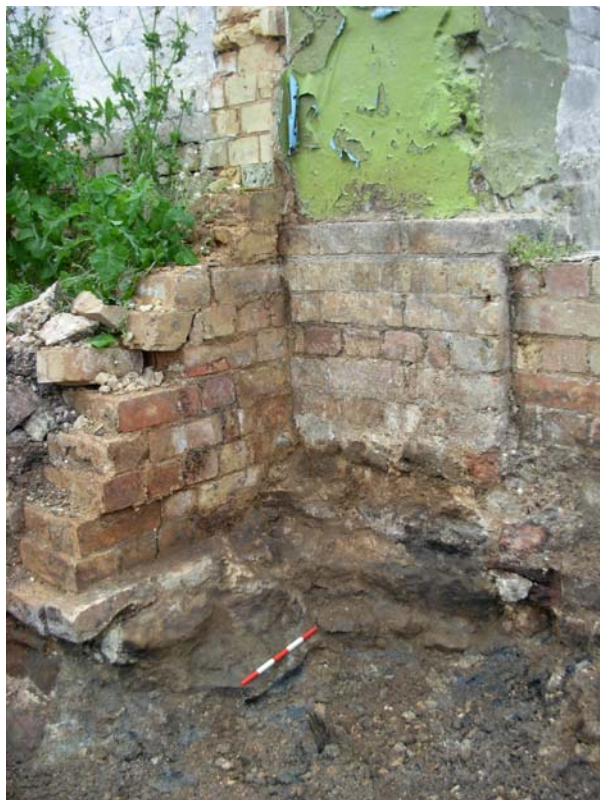
Image 11: Ironstone wall footings of ancillary building, exposed beneath later brick walls situated at SE corner of the Mill Building. Scale 25cm in 5cm divisions.
