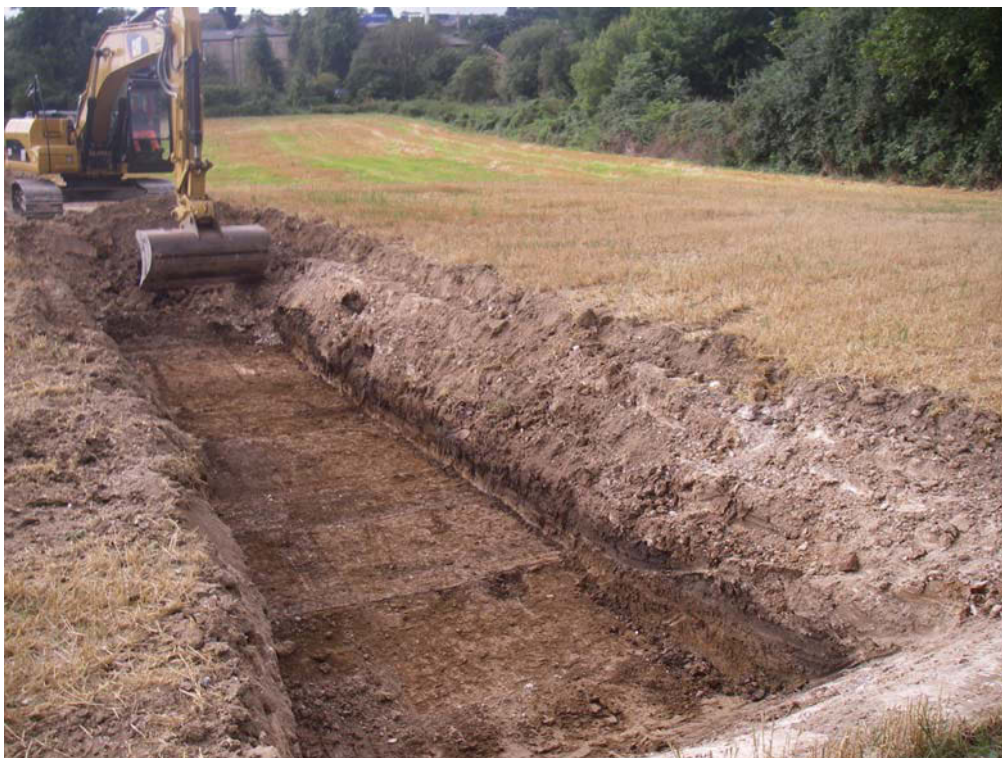
Figure 22: Depth of demolition layers in north-western part of site (start of machining)
