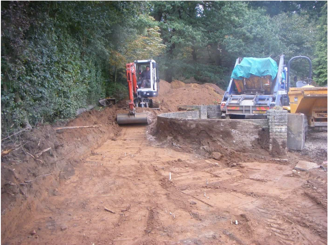
Figure 3: Ground reduction in northern part of site behind retaining wall of raised garden
