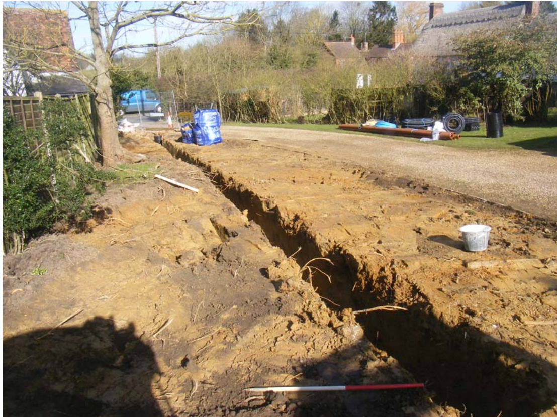
Figure 3: Service trench excavated in the area of previously removed landscaping deposit, looking north
