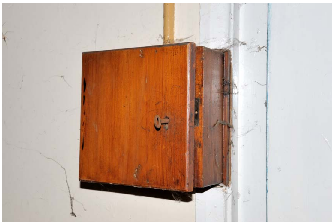
Image 25: Interior: detail of light switches next to south door
