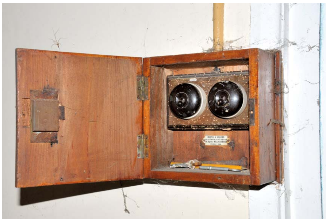
Image 26: Interior: detail of light switches next to south door
