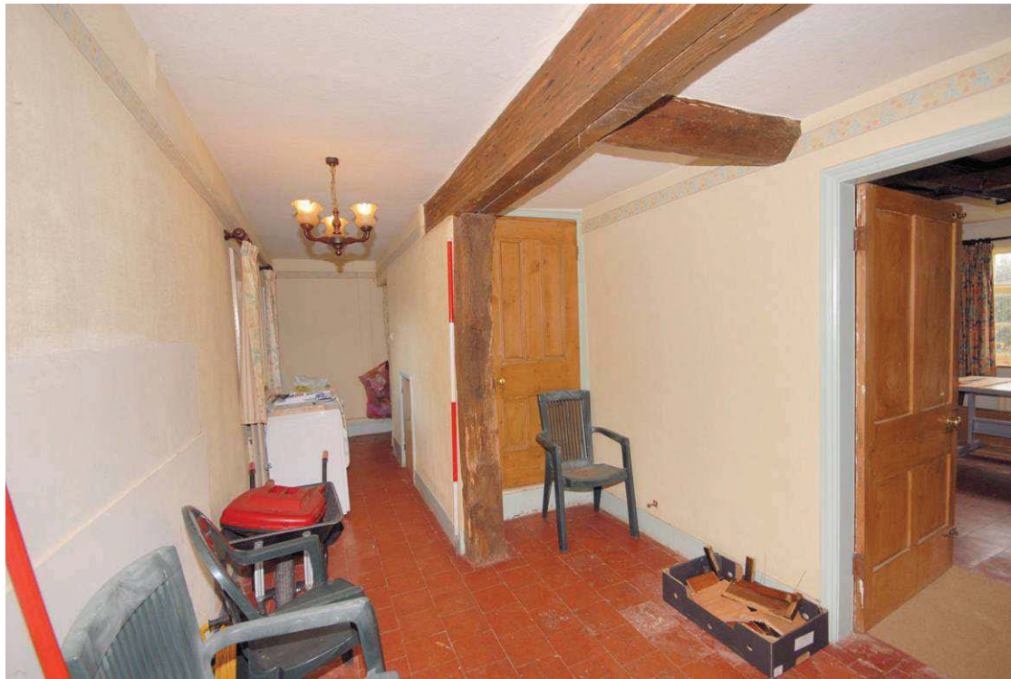
Image 23: Ground floor hall Looking east with door to room 4 at right hand side of image
