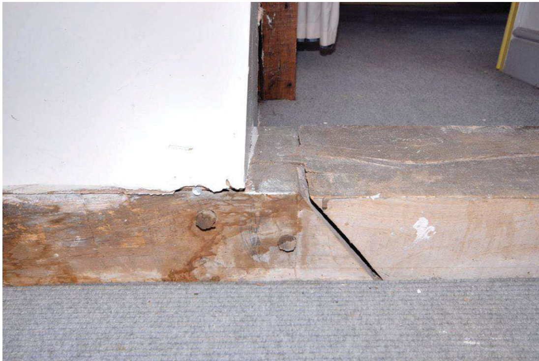
Image 44: Second floor room 3: detail of scarf joint in wall plate View looking east from inside roof space shown in following image
