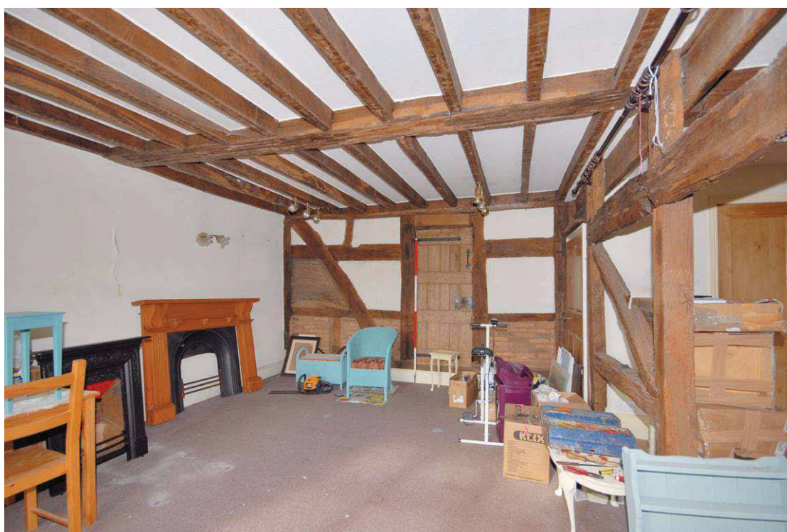
Image 20: Ground floor room 5 Looking north with timber partition to room 4 on the right hand side.
