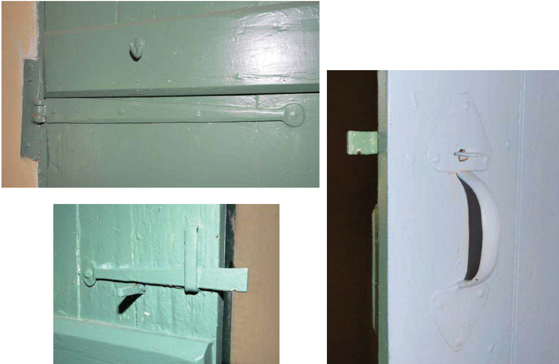
Image 41: Second floor room 2: details of door fittings Strap hinge with rounded terminal and door handle with large leaf-shaped ends.
