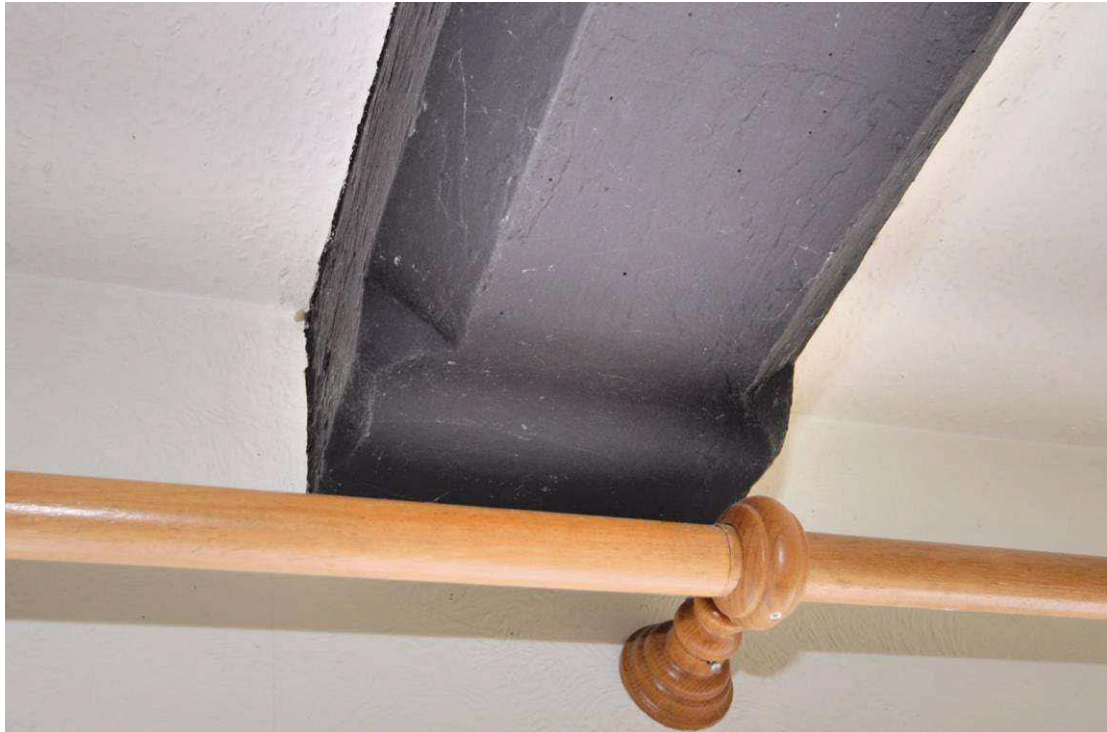
Image 26: First floor: detail of stop on chamfered beam Western end of the beam which is visible in the corridor adjacent to room 1
