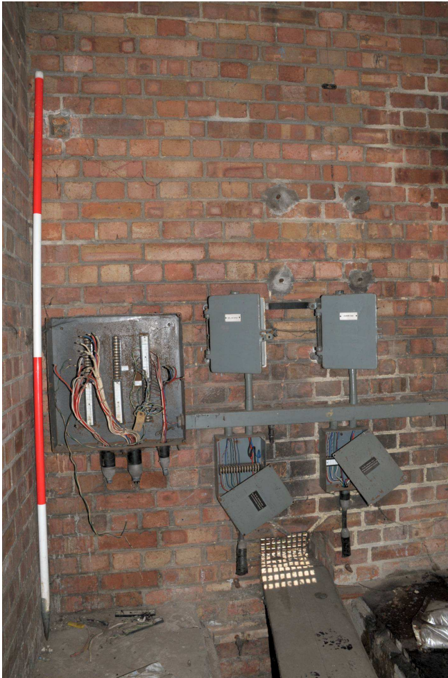
Image 25: Interior detail: Electrical equipment.
