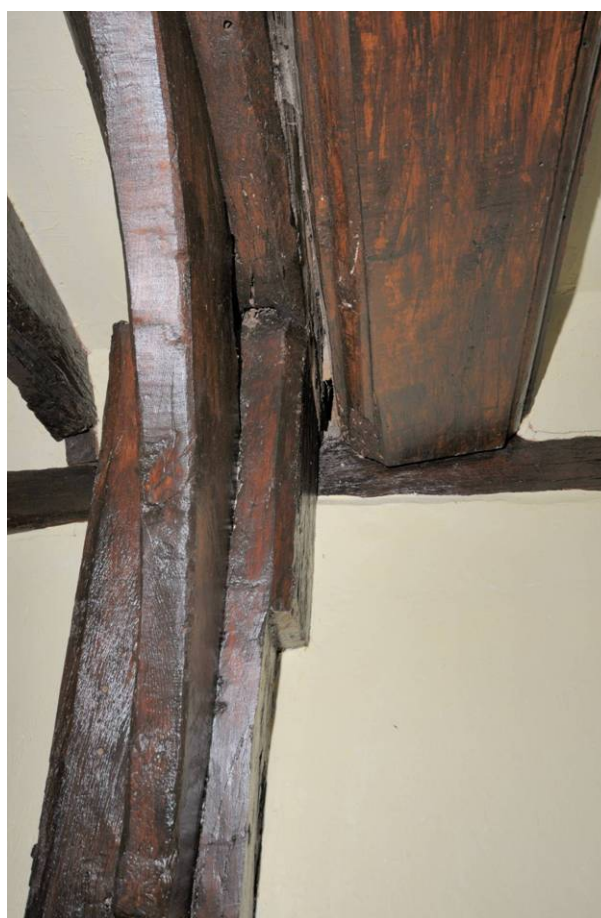
Plate 18: Main range, first floor, south room, frame and chamfered beam Shows frame with arch brace to left and inserted ceiling beam with ovolo chamfer to the right.
