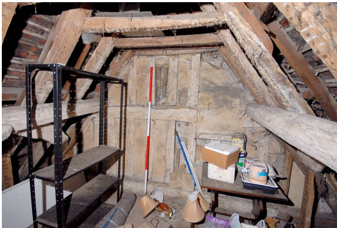
Plate 27: Main range, attic, north bay showing north gable wall. This shows the close studded gable end with a later blocked window where the collar beam has been truncated on the right hand side.
