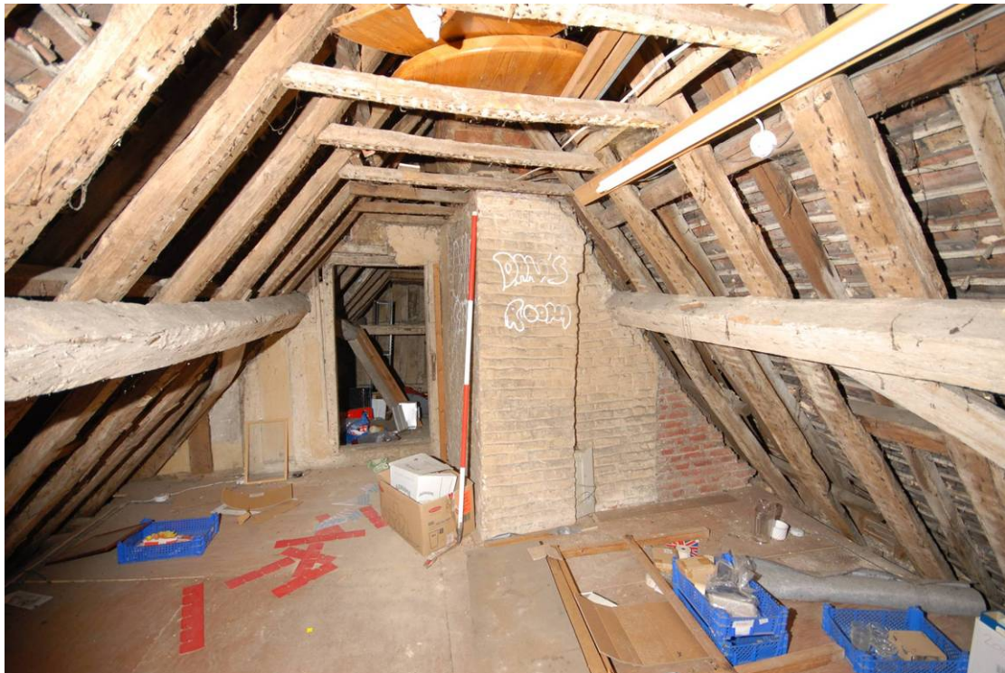
Plate 26: Main range, attic, central bay, looking north Note vertical line in whitewash on chimney stack showing limit of former lath and plaster lining.
