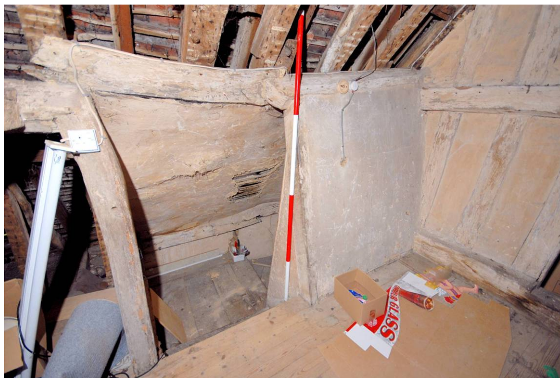
Plate 28: Main range, attic, north bay, showing inserted stair from first floor. The purlin is truncated above the stair and the lath and plaster partition for the stair abuts the original close studded attic partition in the right of the image.
