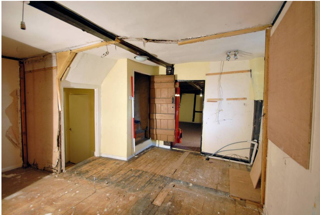
Plate 19: Main range, first floor, north room looking south Shows traces of former room partition visible on ceiling and floor and open door to the attic in centre of image.
