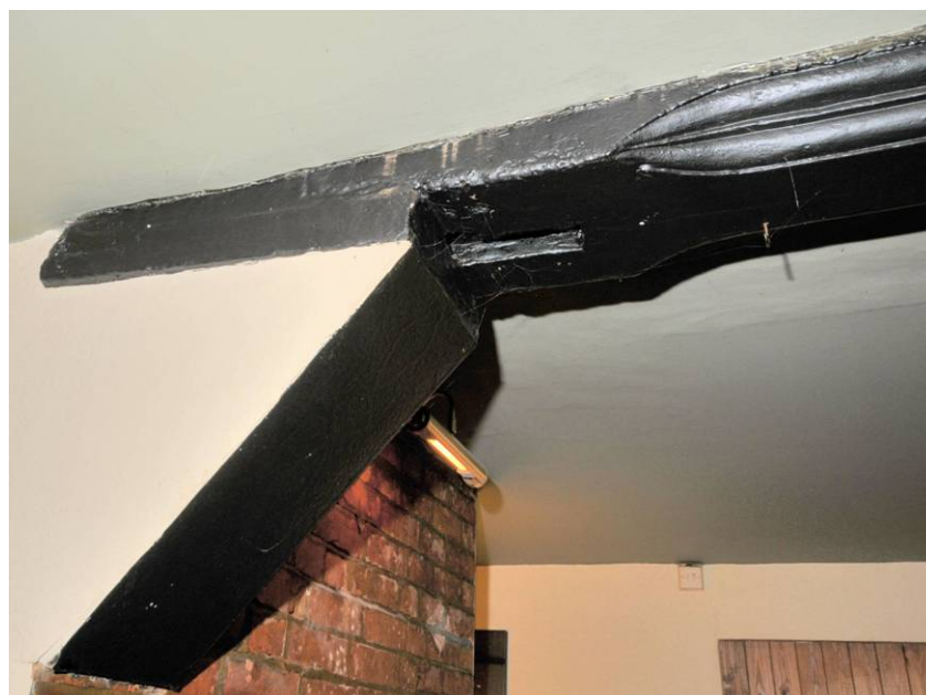
Plate 12: Converging chamfer stop, rear wing, ground floor The end is supported by a modern corbel set in the re-built fireplace
