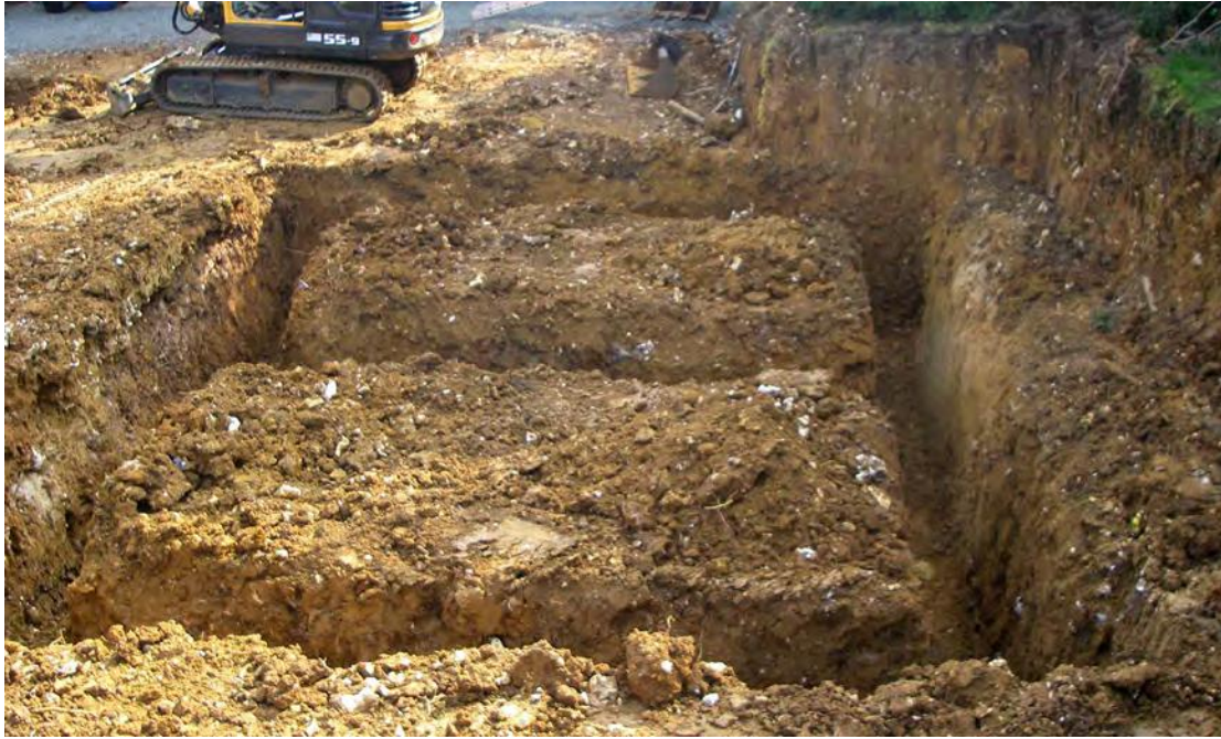
Image 1: General view of excavated footing trenches set within an area of ground reduction. Image is looking towards the house in a north-easterly direction.
