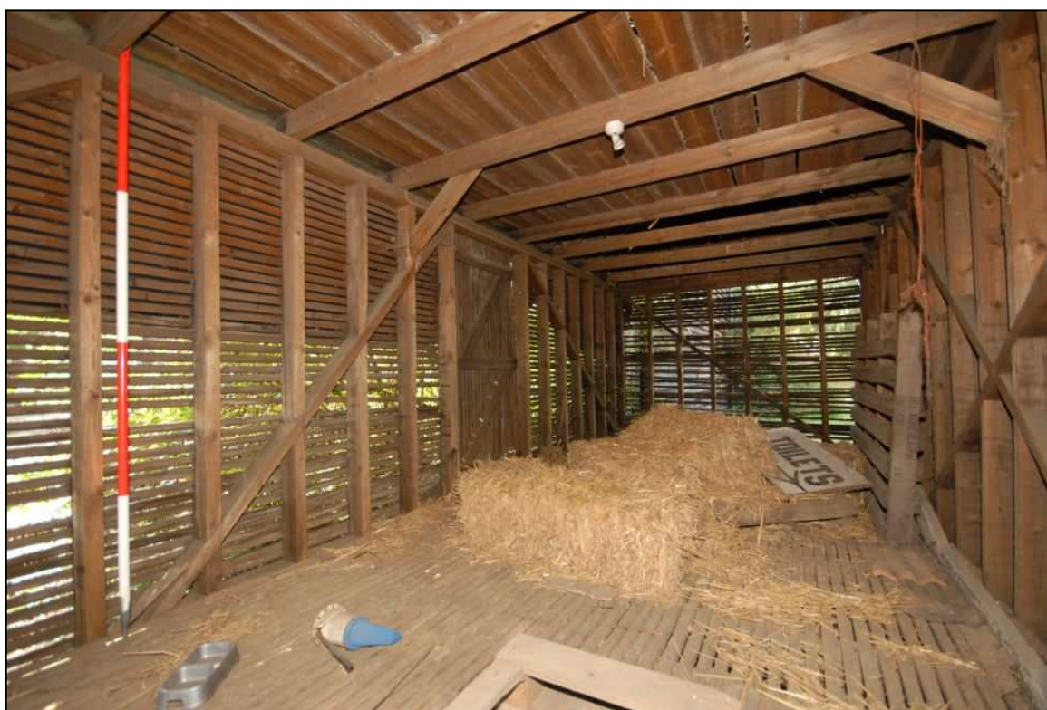
Image 8: Interior view showing the south end and east side walls (scale 2m)
