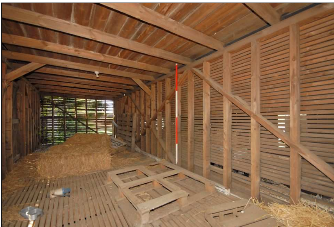
Image 9: Interior view showing the south end and west side walls (scale 2m)
