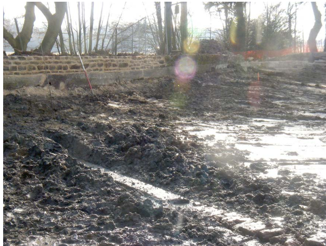
Culvert, training wall of weir in the background, looking south west. Scale 1m
