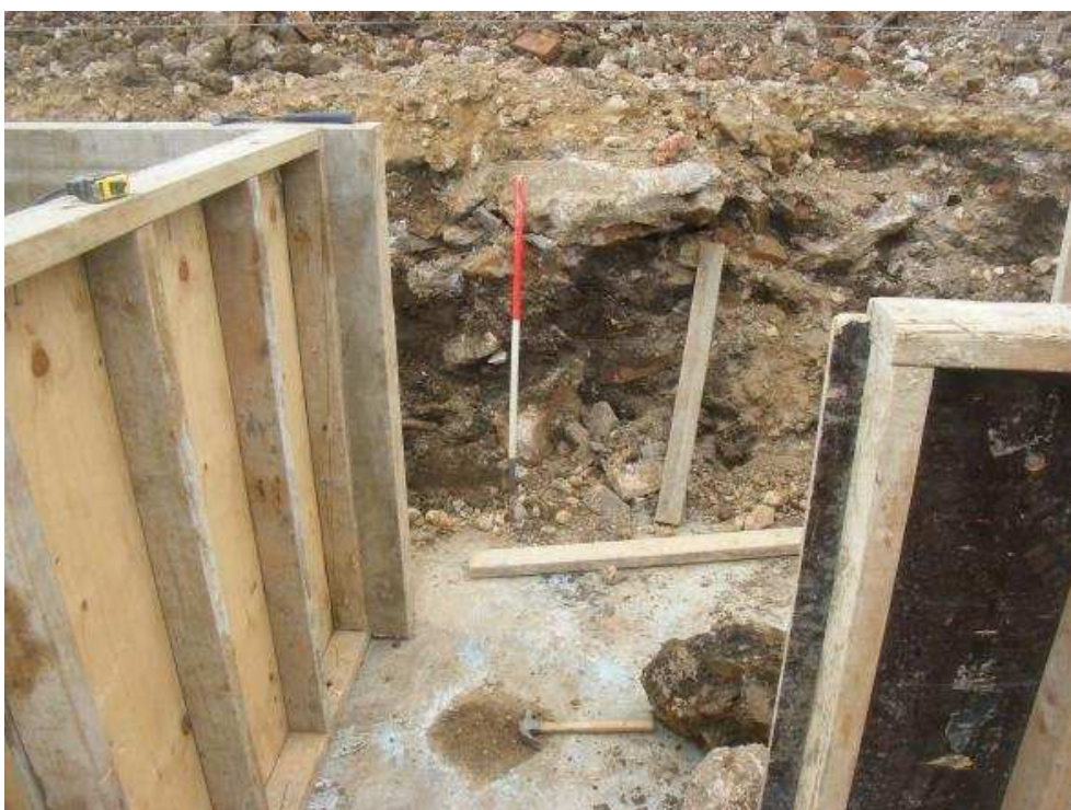
New formwork in place on top of intact blue concrete base of former swimming pool, with the material used to backfill the pool visible in the background
