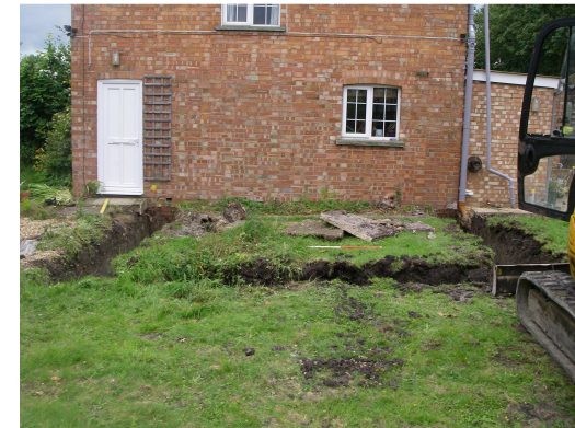
Image 1: General view of footing trench with gable end of West Cottage beyond
