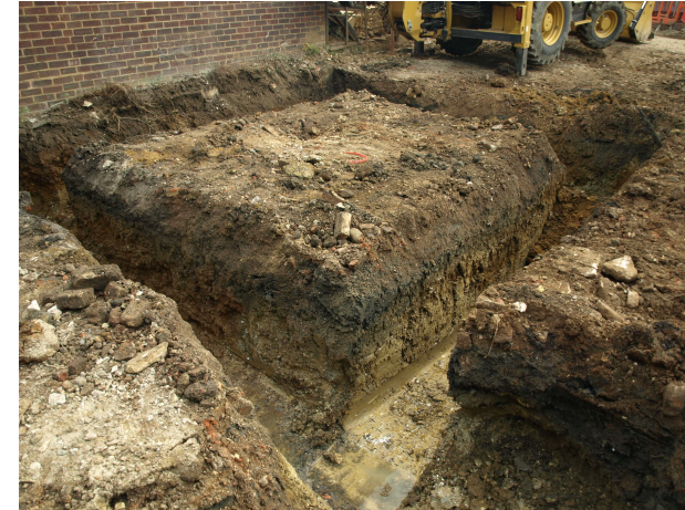
Above: Dark-coloured former farmyard layer (201) observed in foundation trenches beneath concrete slab
