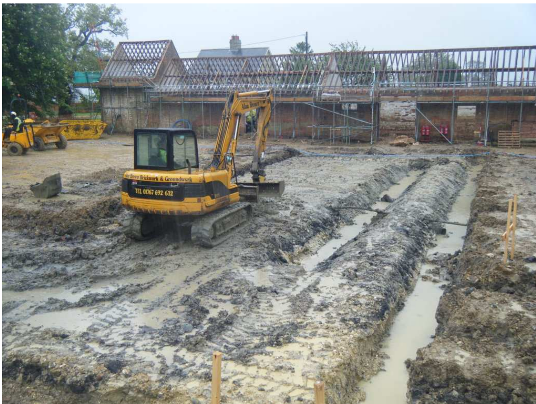
Image 8: Zone E during the construction phase Machining in the west arm of Zone E, showing the completed ground reduction for the floor slabs and partially excavated strip foundation trenches
