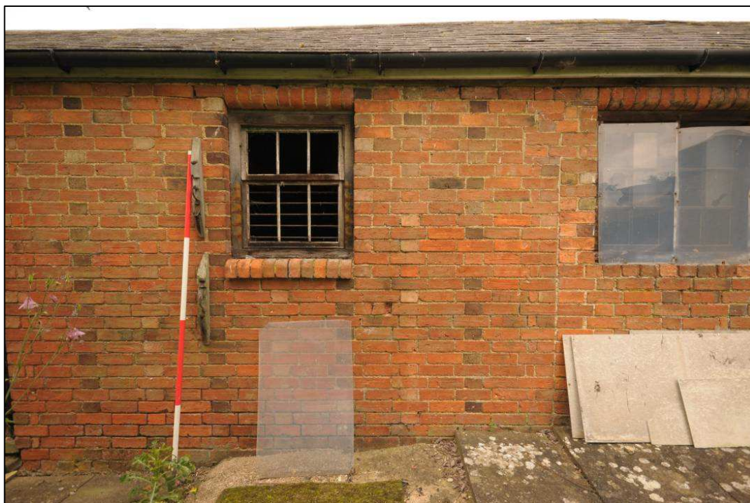
Image 7: West range: showing east wall of stable and tack room (shows straight joint between brickwork of stable and tack room on the right)
