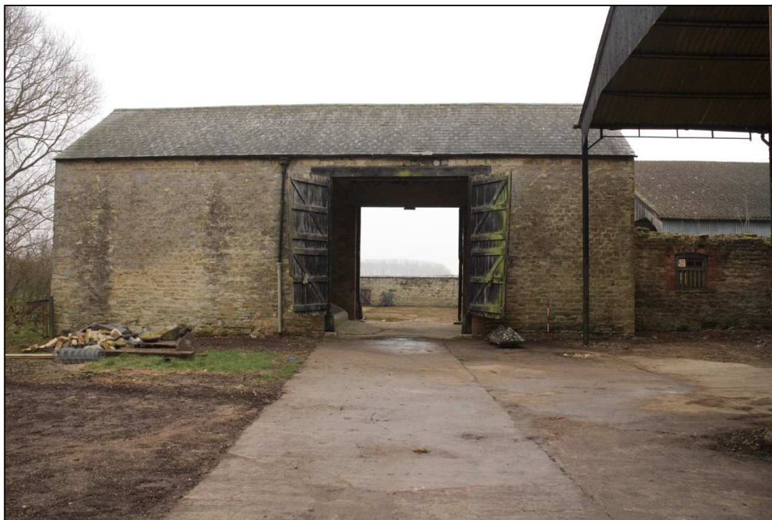
Image 17: North range: C7 Barn: Exterior view of north elevation Shows proportions of barn with longer section to east of doors
