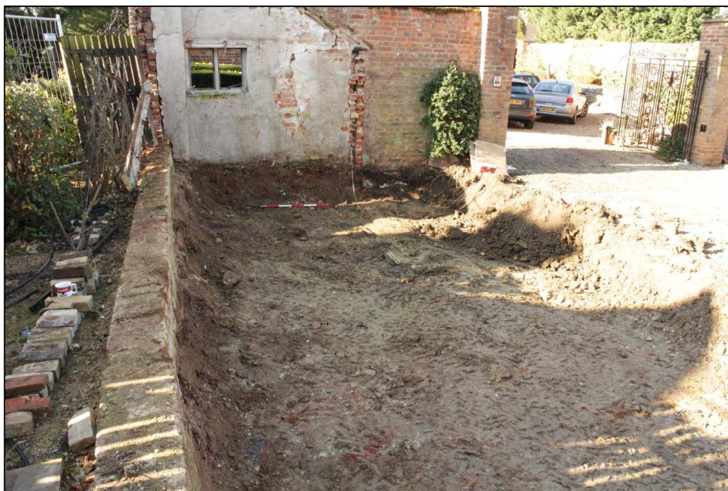
Image 7: Western end of trench (View looking towards west end of trench following completion of machine excavation (scale 1m))
