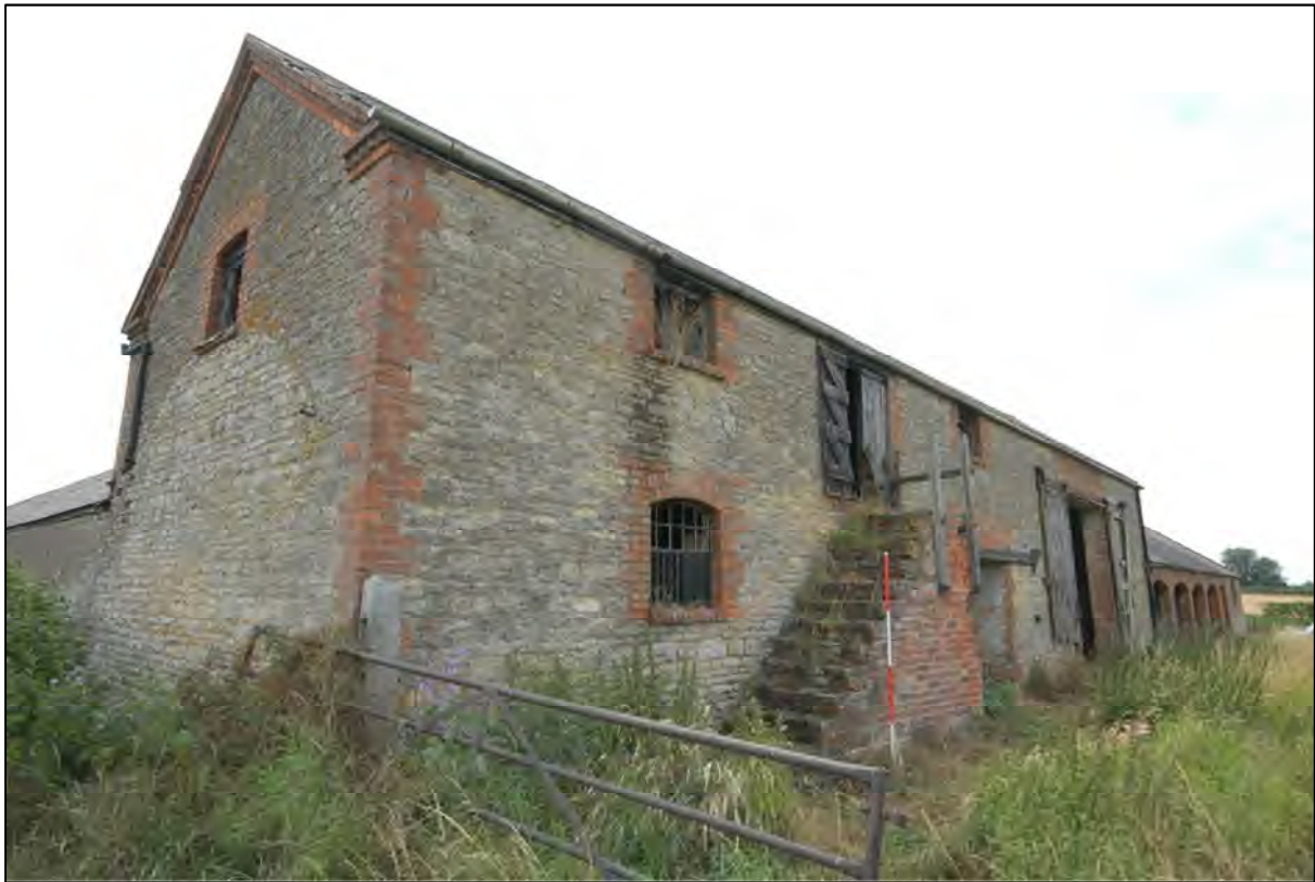
Image 15: Exterior view of north range, looking south-west Showing two-storied section (C5, C6 and C7) in foreground
