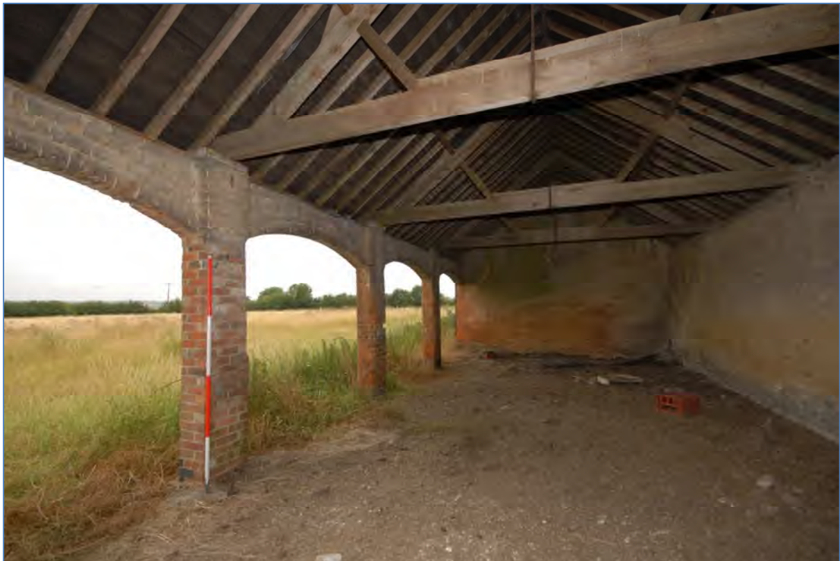
Image 18: Compartment C3, view looking east Showing brick piers and arches supporting open side to the north
