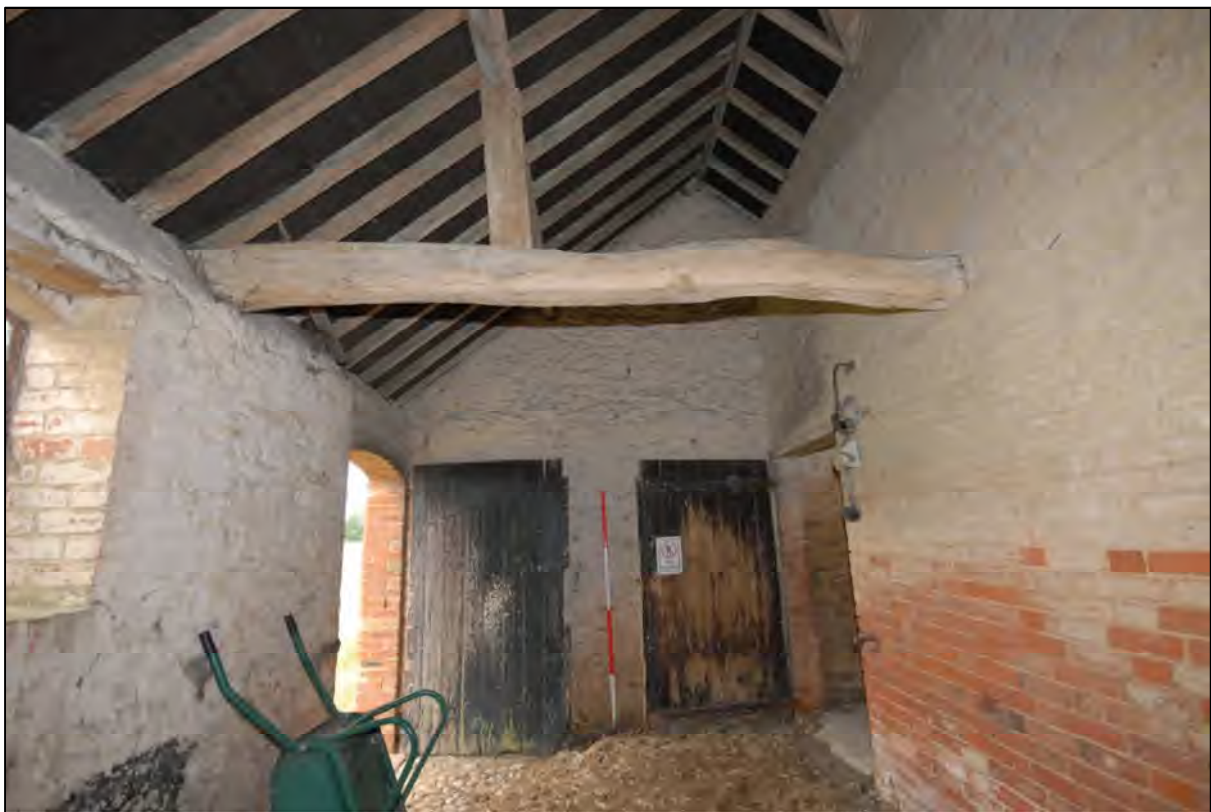
Image 14: Compartment C2, view looking east Showing exterior door in north wall and interior door to C1 at right
