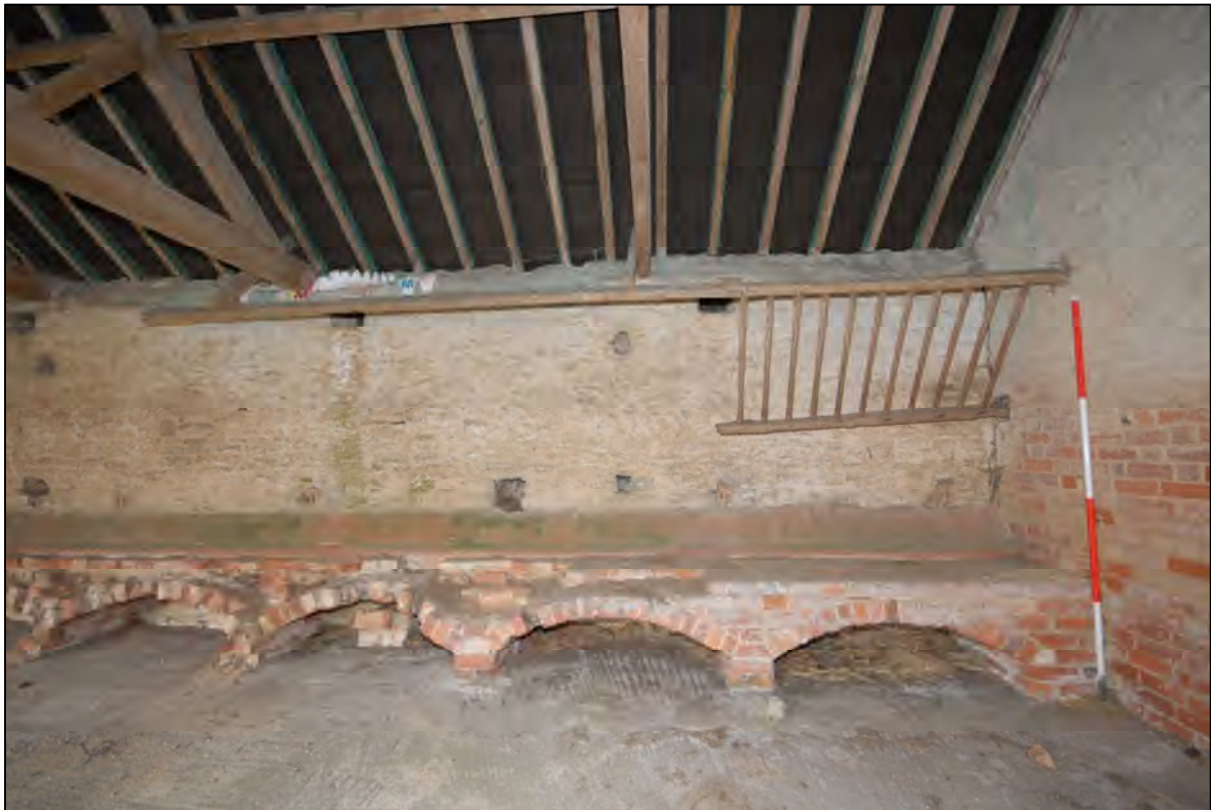
Image 13: Compartment C1, detail of brick trough and hay rack Shows remains of wooden hay rack and brick trough at north end of C1
