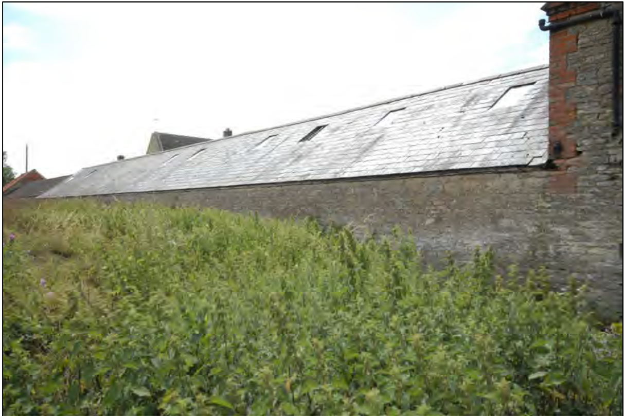
Image 27: Exterior view of east range, looking south-west Showing the outward-facing east elevation
