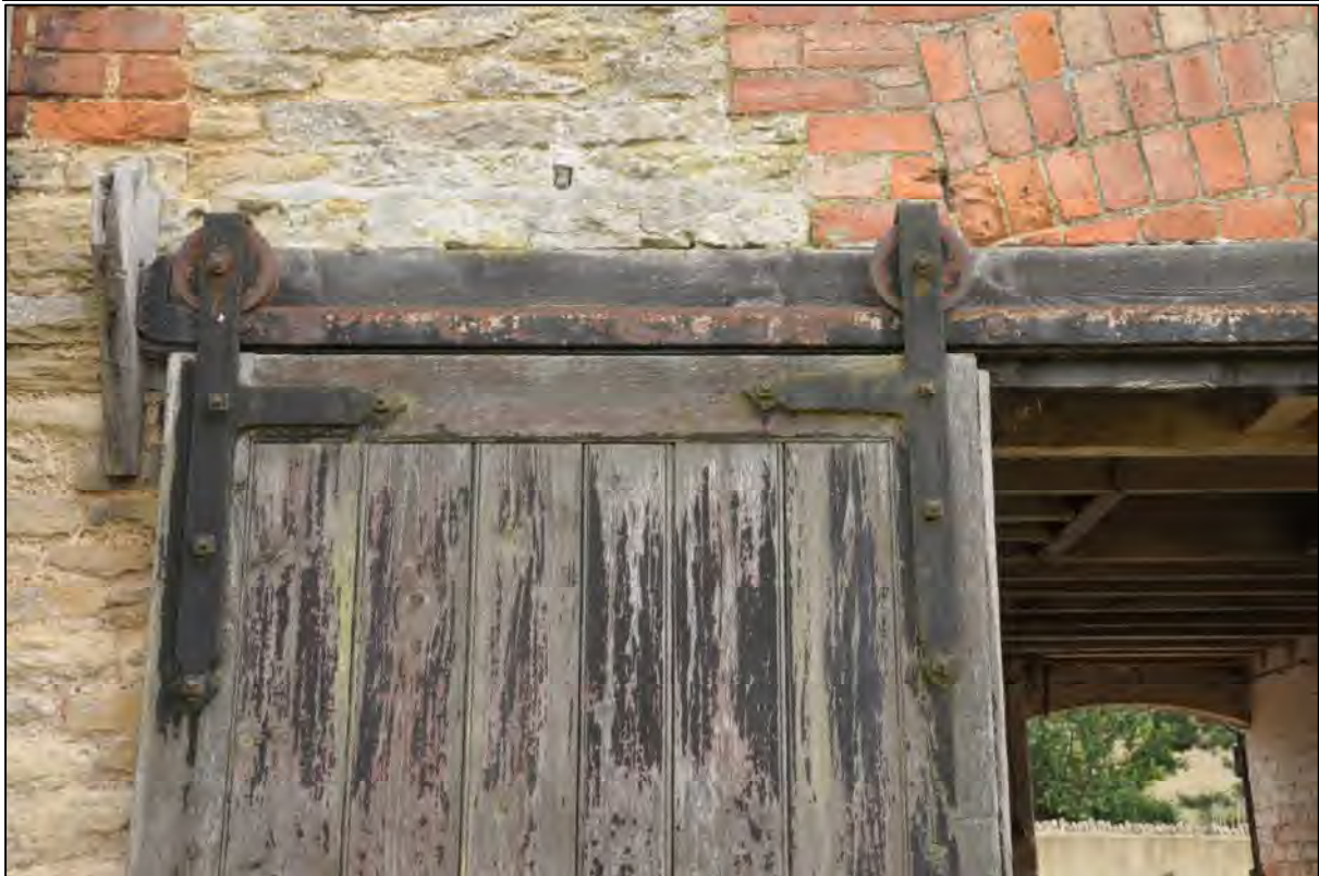
Image 5: Exterior sliding door on the north range Shows fittings of the door to compartment C4
