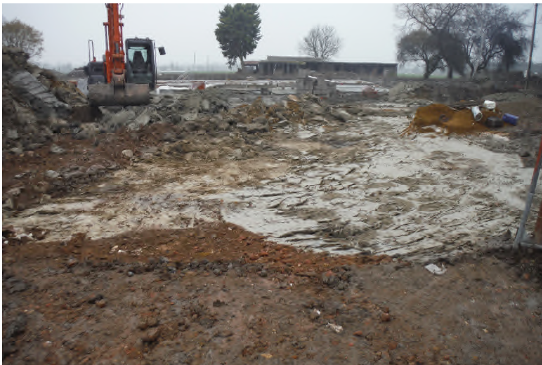
Image 3: View into the site from vicinity of Higham Gobion Road, looking towards the partly constructed basement in the middle distance and an old farm building beyond.
