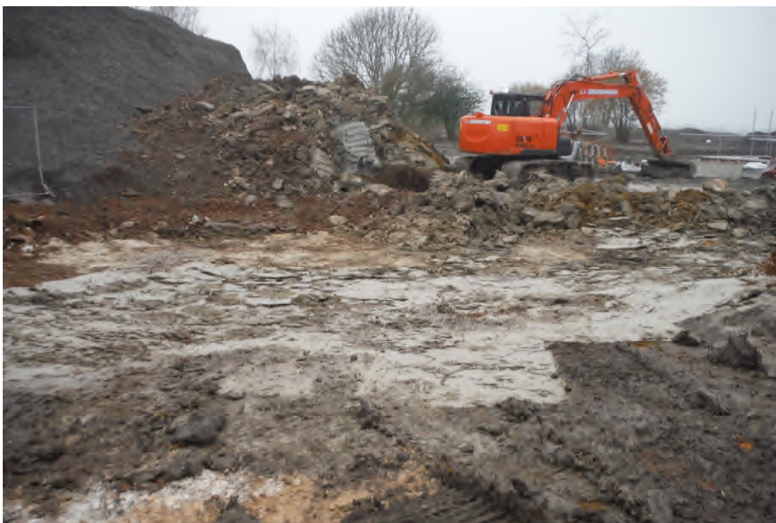
Image 4: Stripping of the main part of the access road and turning area, to the level of the undisturbed geological strata.
