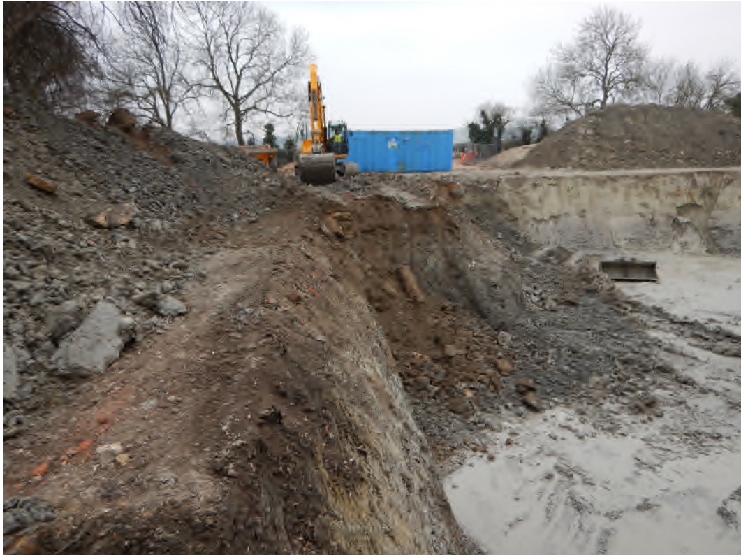
Image 1: Stripping of the footprint of the new dwelling. The large cavity to the right of the image is part of the basement already stripped to formation level.
