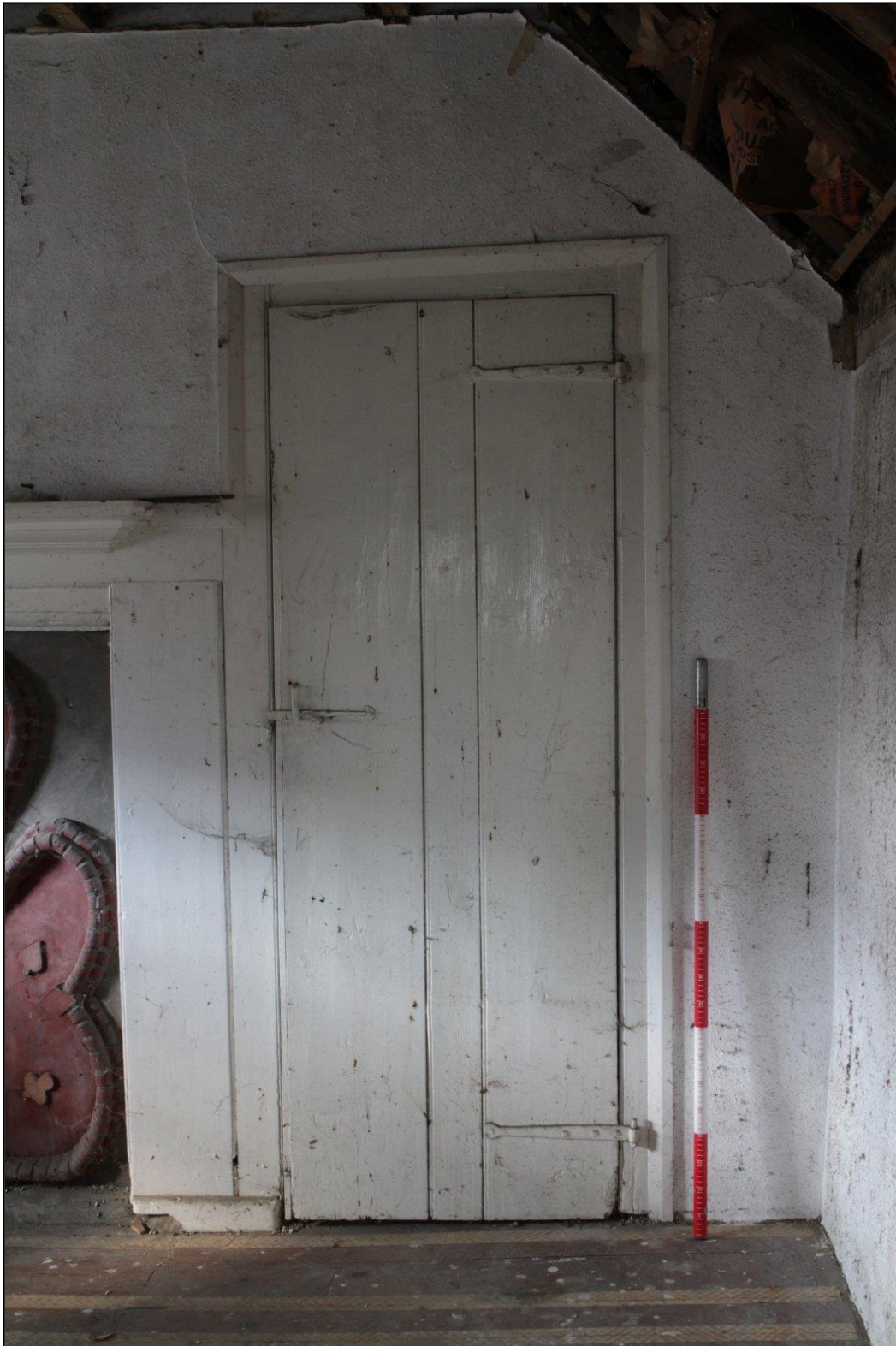
Image 19: Room F1, detail of door next to the fireplace Shows three-plank door with strap hinges on pintles (Scale 1m)
