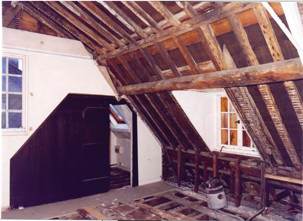
Plate 23: Attic floor, northwest corner, showing landing to secondary stairs and dormer window
