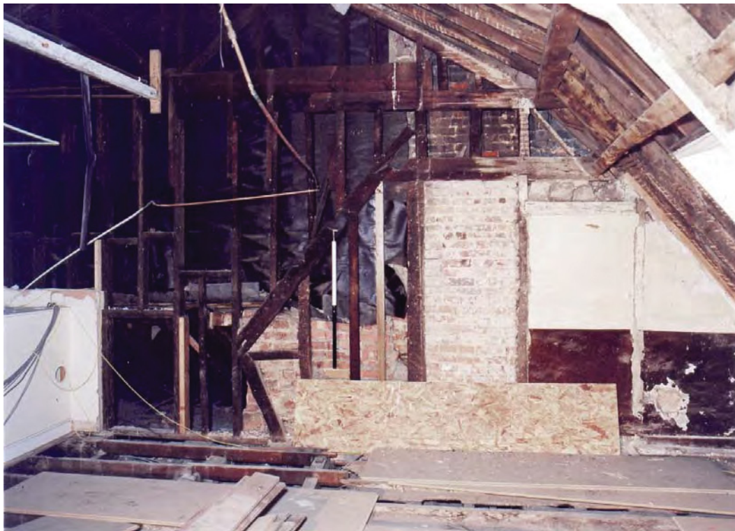
Plate 24: Attic floor, southeast corner, showing framing of 18 th century gable incorporated into 19 th century mansard roof structure
