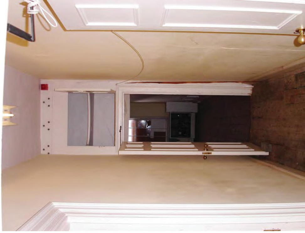
Plate 17: First floor, corridor between rooms G6 and G8, showing cupboard above doorway
