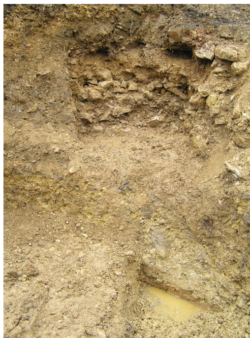
Photograph 11: Investigation of ground paddle channel and form of canal in Trench 4. Two narrow 'steps' or 'shoulders' are clearly visible in the canal lining.
