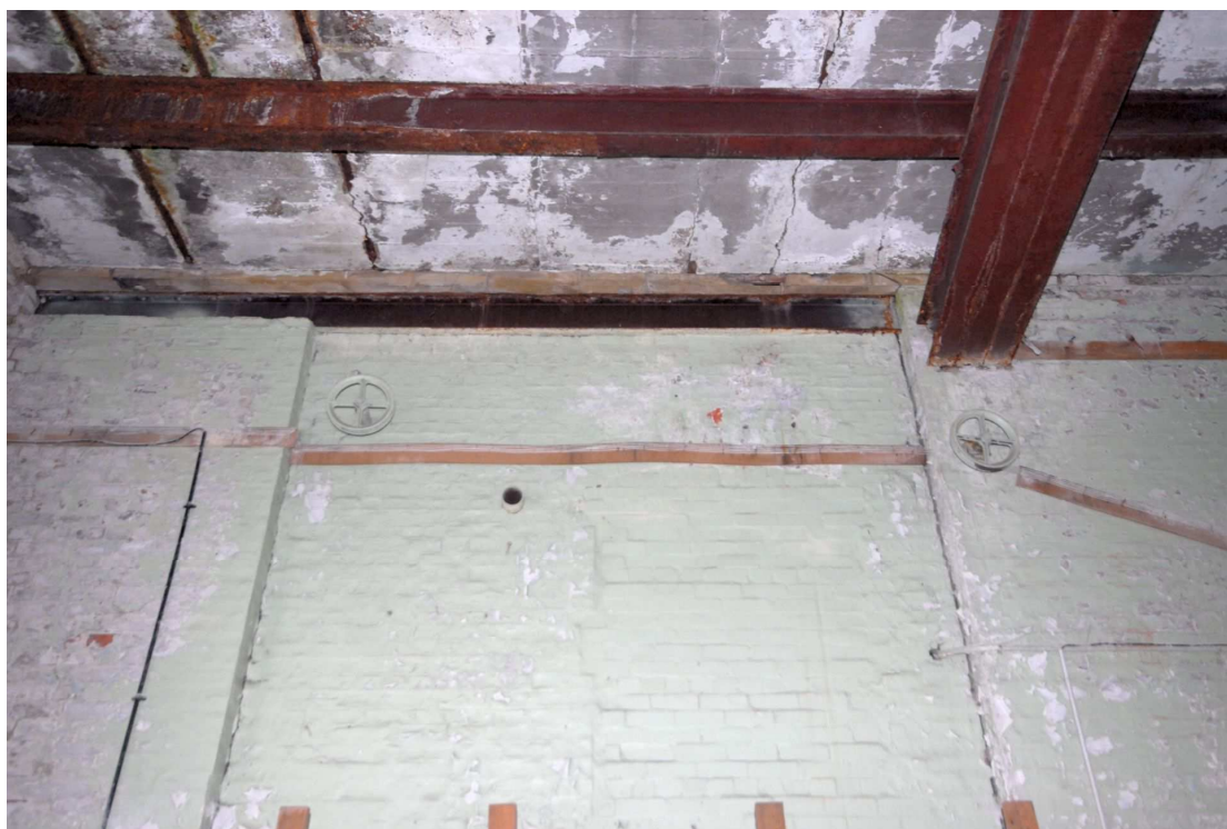
Figure 13: Wheels for possible rope fittings to operate ventilation shafts at southern wall of boiler house (not original ceiling).
