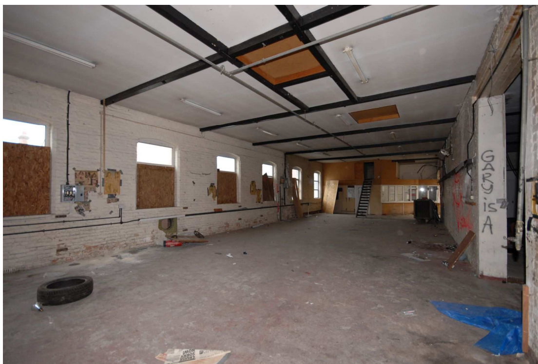
Figure 17: Former “Sorting and Packing Room”. Image taken in same direction as historical photograph in Figure 16.
