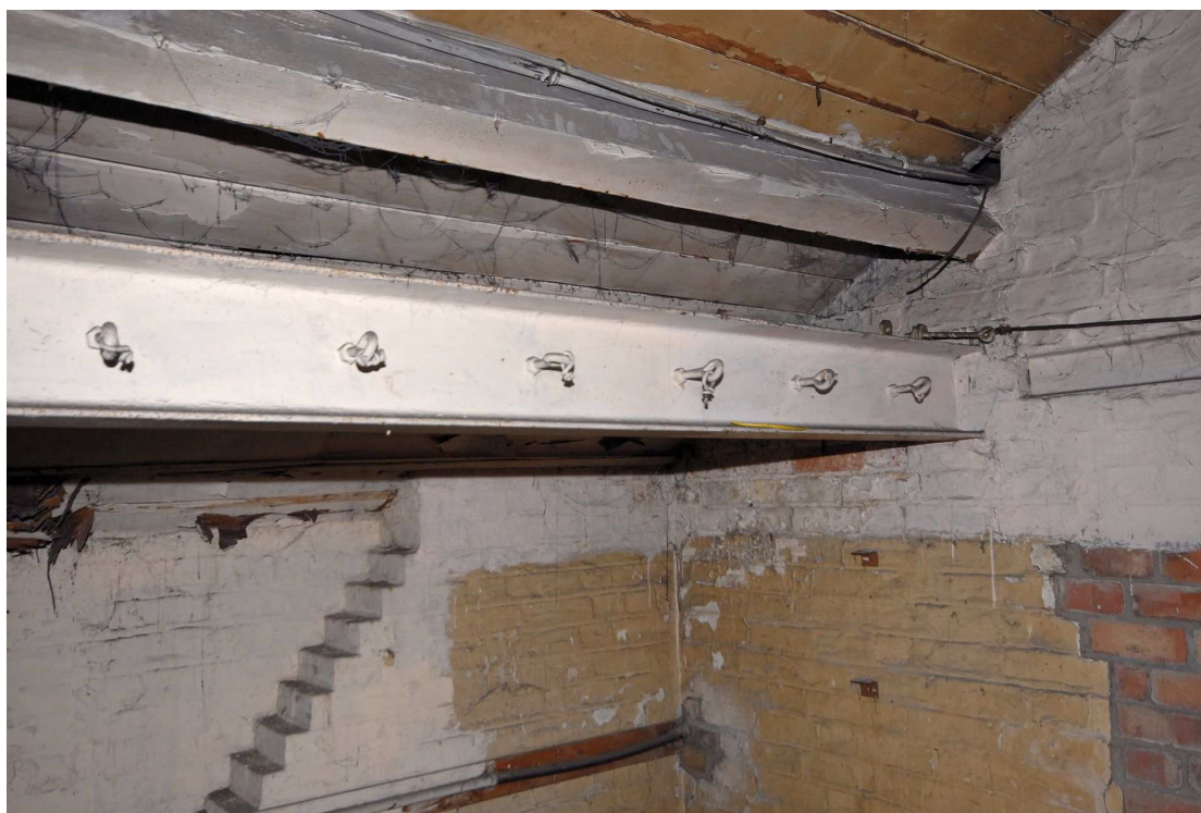
Figure 15: Hooks in area of former “Drying Closets” for rope or wire attachments.
