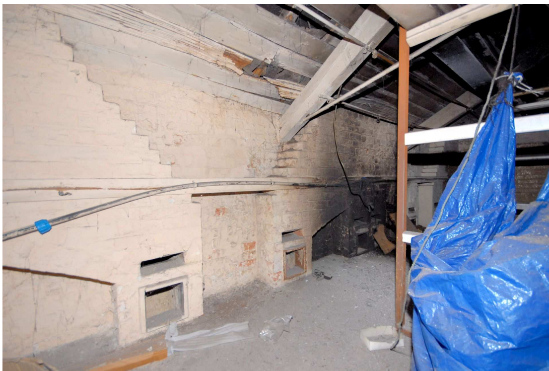
Figure 14: Flues in area of former “Drying Closets”, sharing wall with boiler room.
