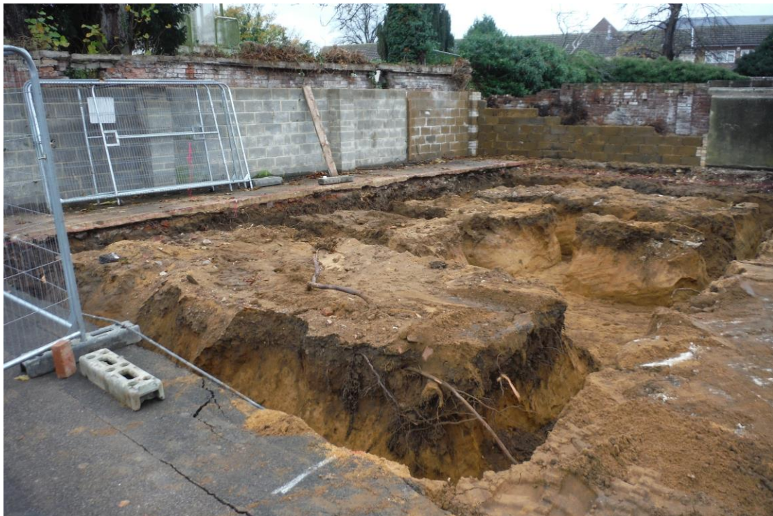
Figure 4: Site of garages following demolition and excavation of new foundation trenches (looking north-west)
