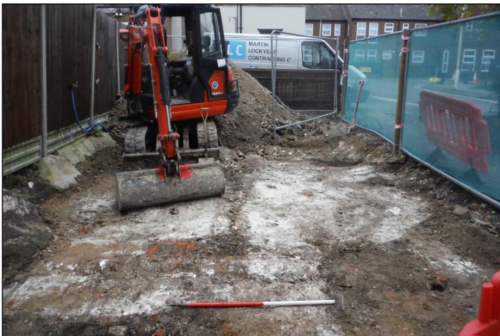
Image 4: South-western part of the lower terrace, with overburden removed, showing modern rectangular pit [10] to bottom right of image, modern service and circular tree-planting pit [11] (Scale 1m in 50cm divisions)
