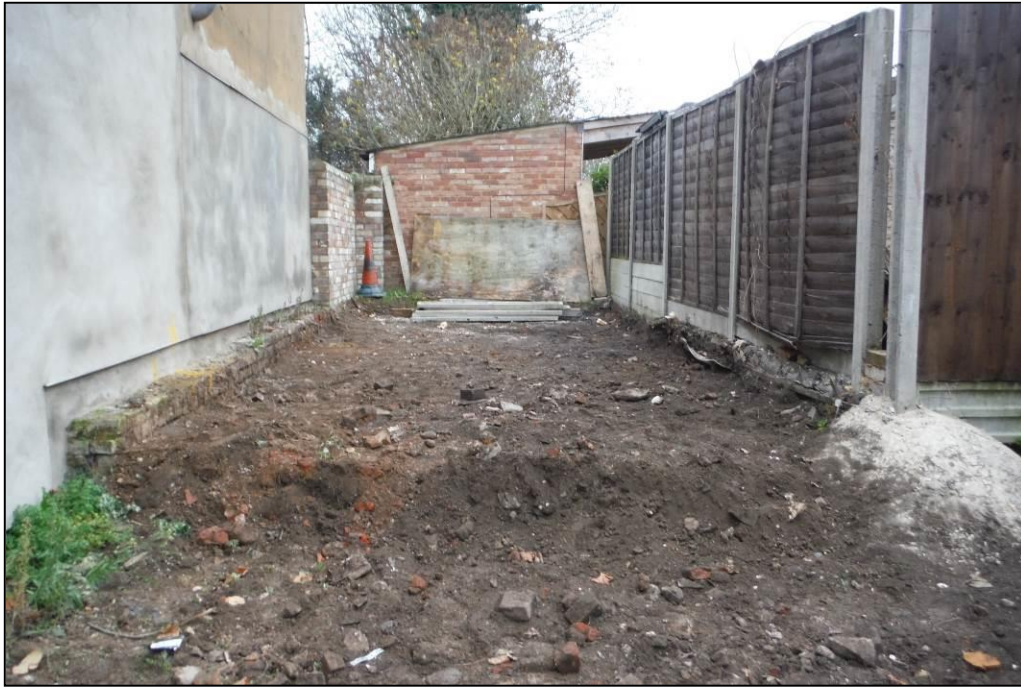
Image 1: Pre-excitation view of garden area of site, looking south-east, showing the height difference between street frontage and the higher ground to the rear of the plot
