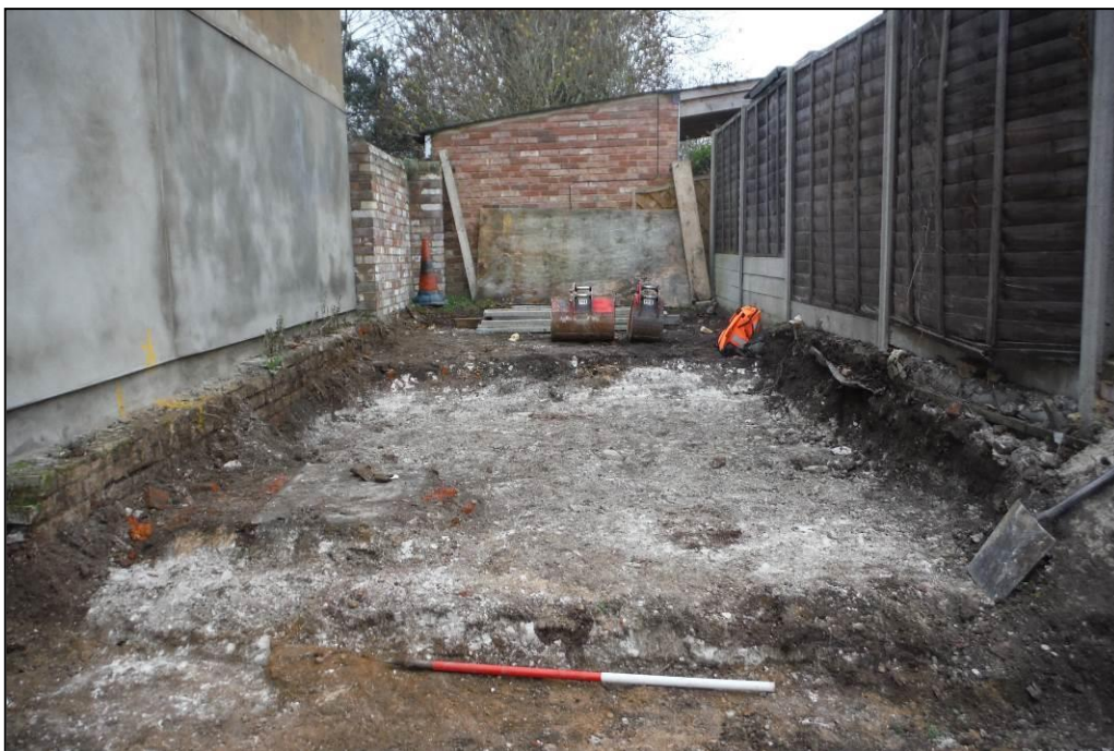
Image 2: Stripping of garden area to the rear of the plot, looking south-east from the street frontage, showing the chalk terrace with foundation trench [7] at extreme left of image and manhole and associated service trench to lower left (Scale 1m in 50cm divisions)
