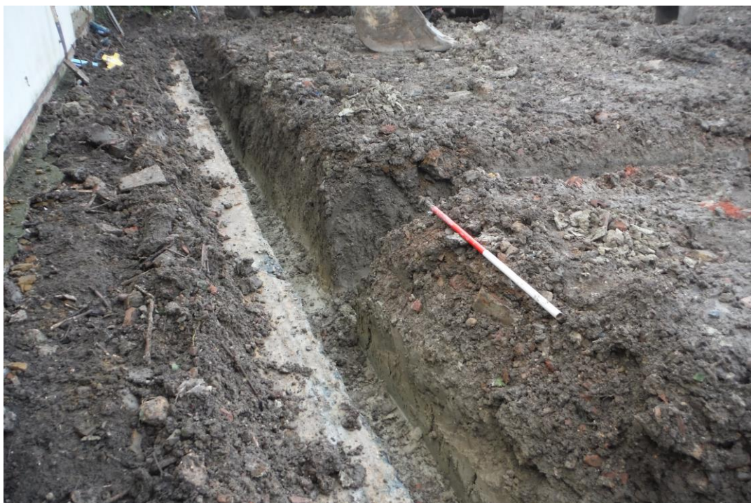
Image 3: Looking southwards along the eastern wall footing trench, which shows extensive dark layer (8) getting thicker to the south, away from the camera. Scale 1m in 50cm divisions.
