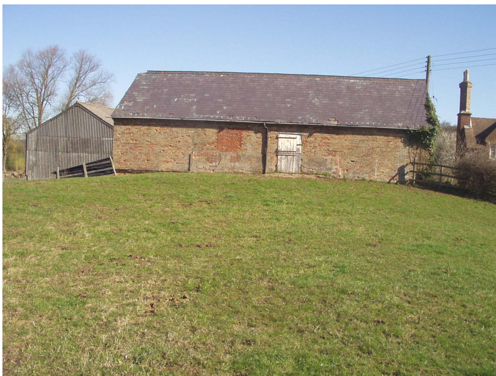
Image 6: View of southern façade of mill building from bottom of ramp (D). The white door is a later insertion; one of several visible alterations to the building.
