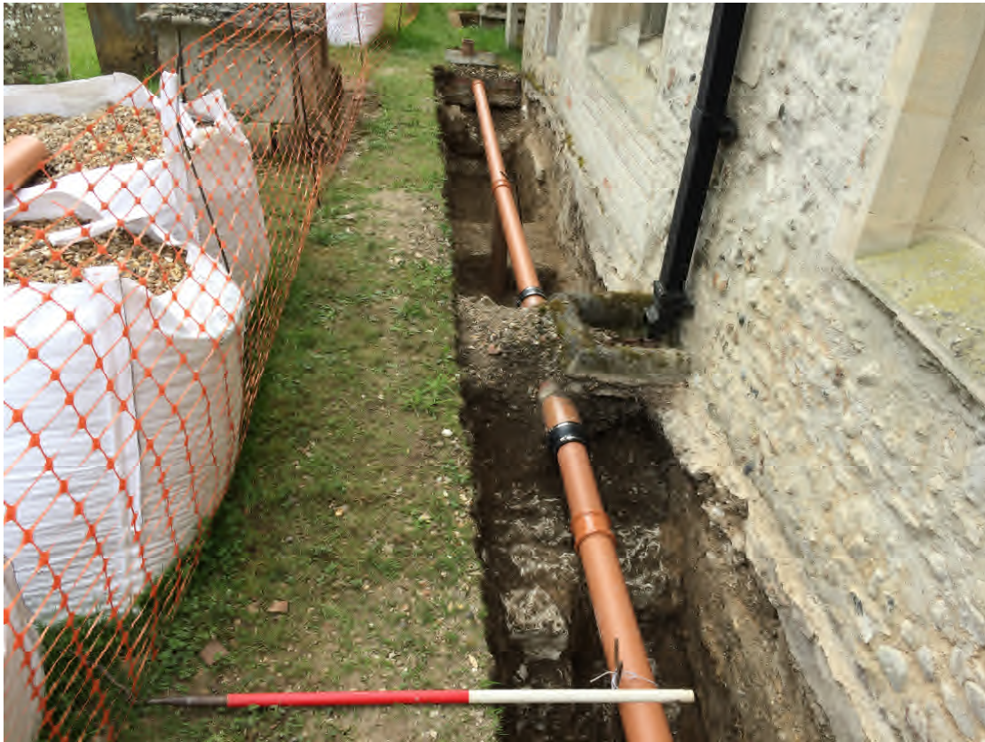
Plate 7: Trench 6 – demolished chapel foundations (611) in foreground and at end of trench. Stone floor remnant (612) towards centre. (1m scale)
