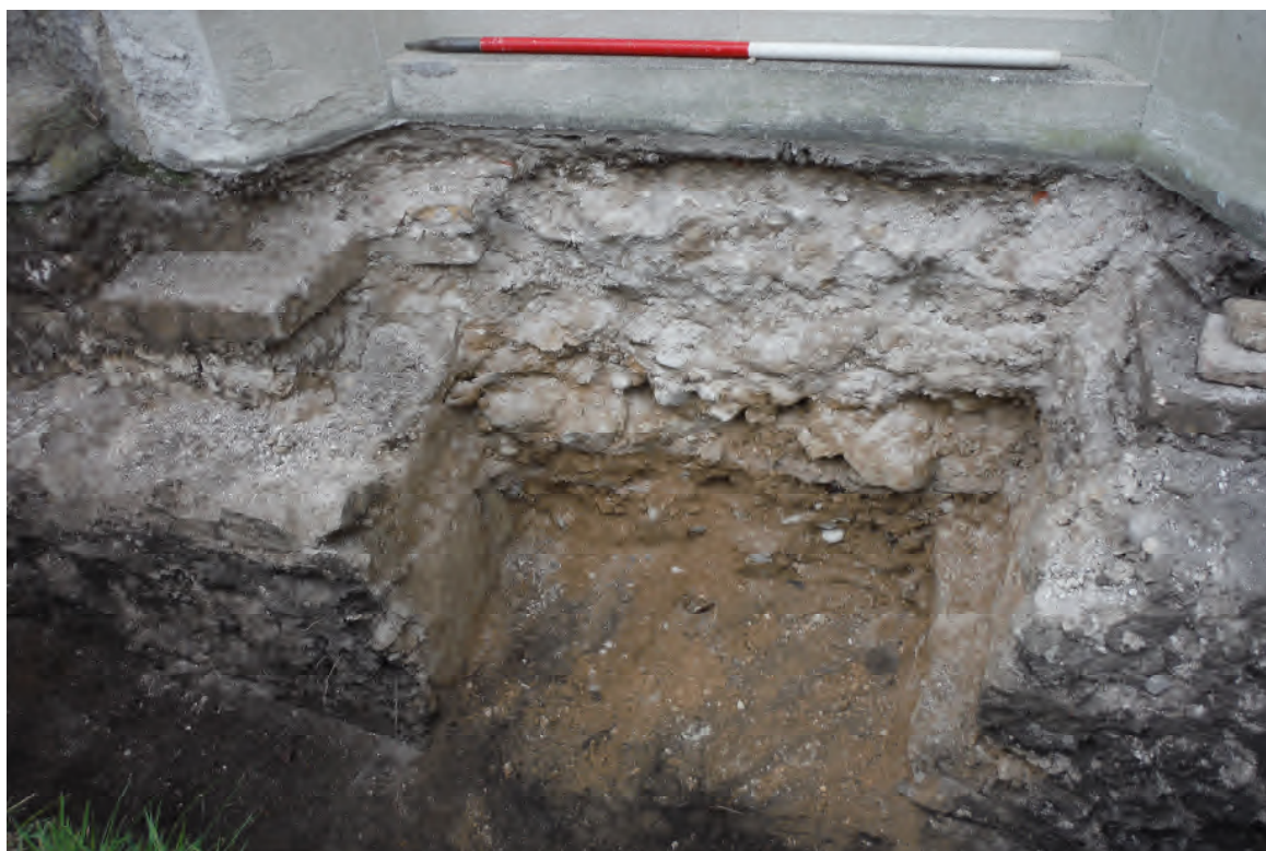
Plate 6: Trench 5 – tower foundation (503) with gap indicating location of former west door (1m scale)
