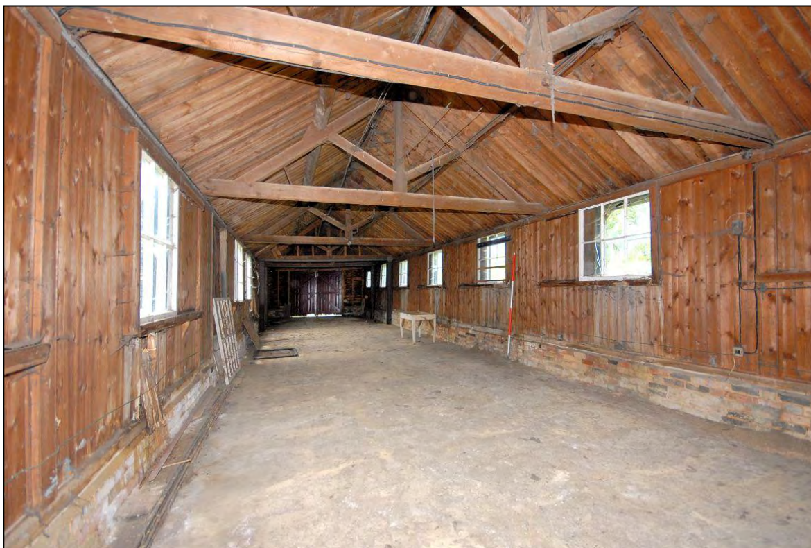
Image 13: West range, south compartment, looking south Looking towards double doors at south end of range (Scale 2m)
