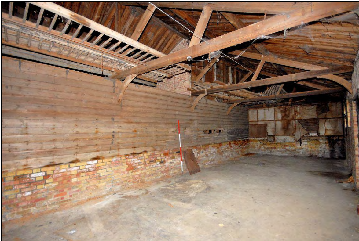
Image 23: Shelter sheds, south shed, looking north-east Shows spine wall with brick sill and plank partition (Scale 2m)
