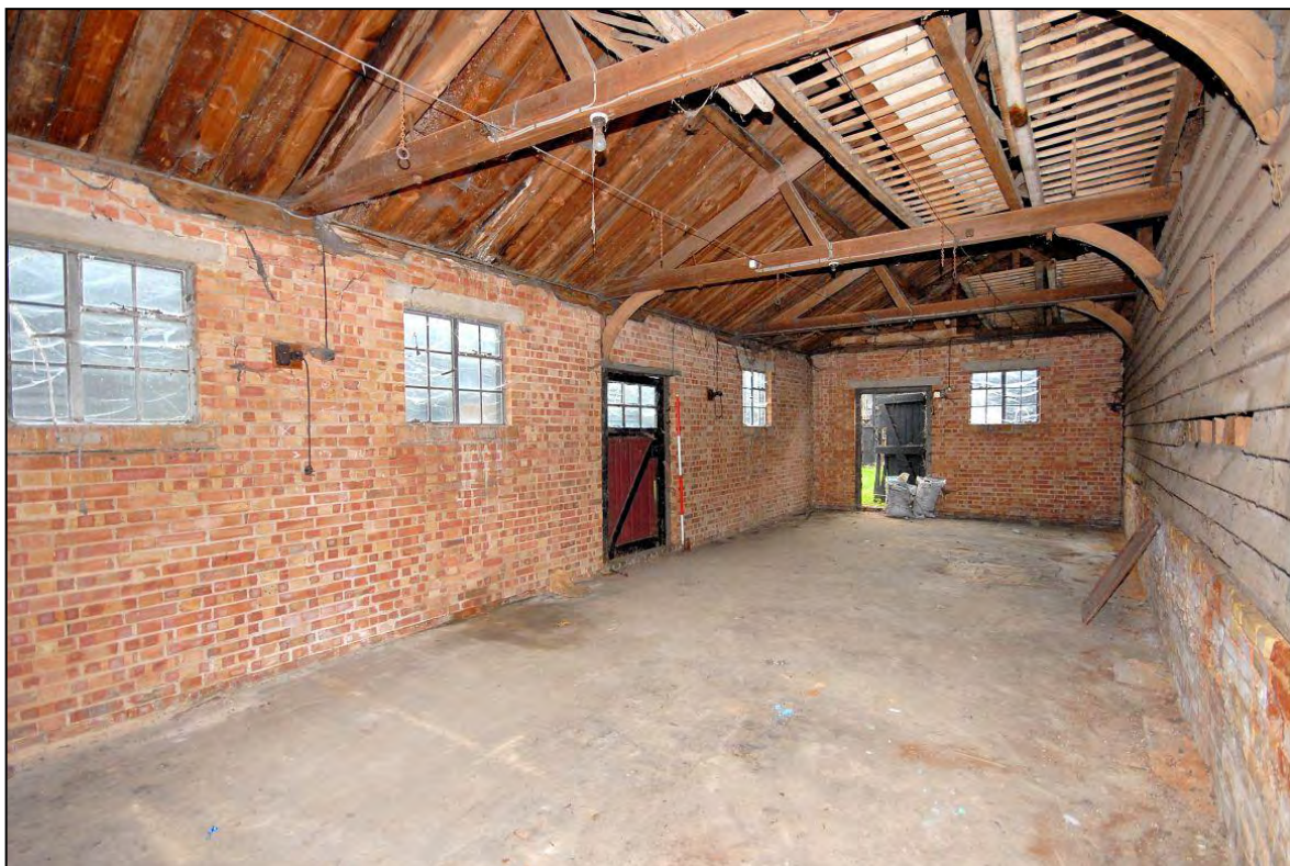
Image 24: Shelter sheds, south shed, looking south-west Shows inserted exterior walls in Fletton brick with metal-framed windows (Scale 2m)
