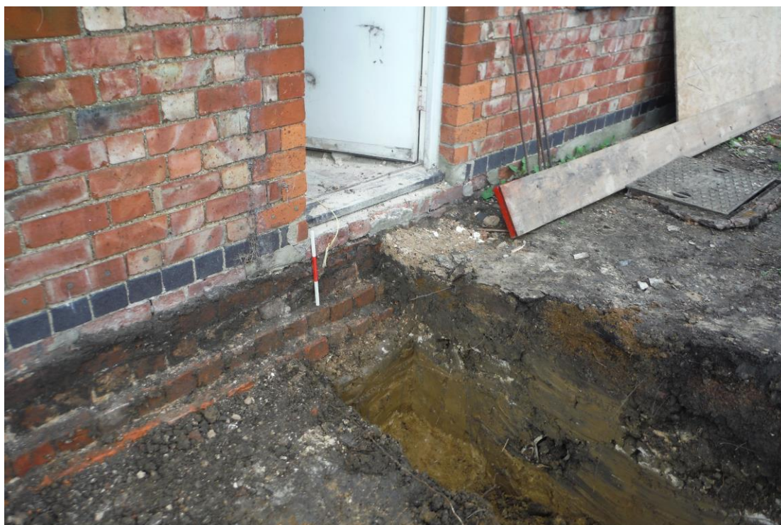
Image 3: NW area of footing trench showing the two sequential drains, with the earlier example [06] parallel to the northern edge of the footing trench, whilst the later example [08] crosses the earlier drain at right angles, truncating it. Scale 0.3m in 10cm divisions.
