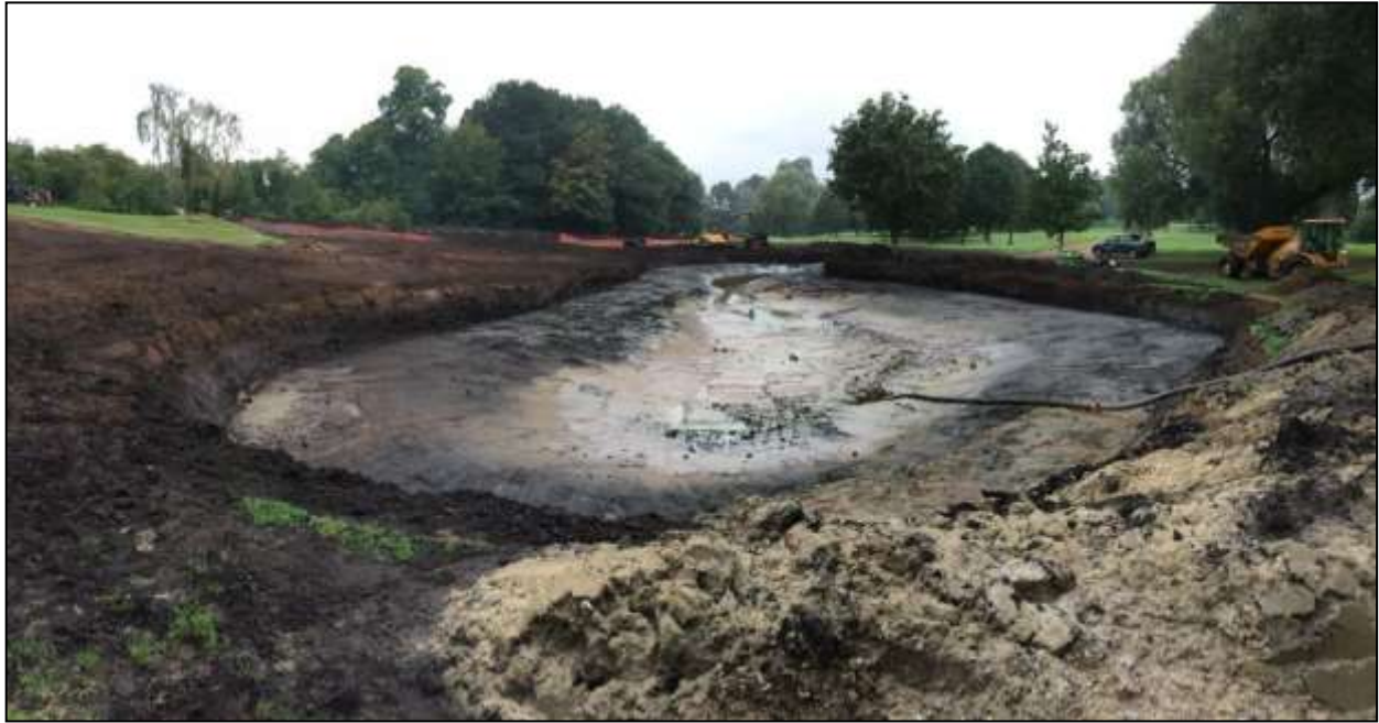
Plate 7: View of the fully excavated new pond in Area B, looking south-west
