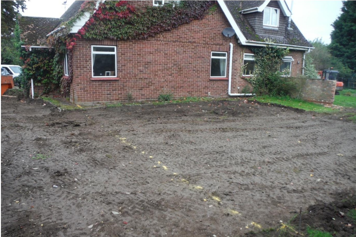
Image 1: General view of footprint of eastern extension, following removal of the turf
