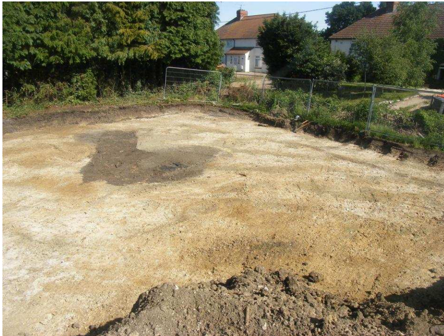
Figure 5: The top of the well and backfilled trial trench after stripping open area for excavation (looking north-west)
