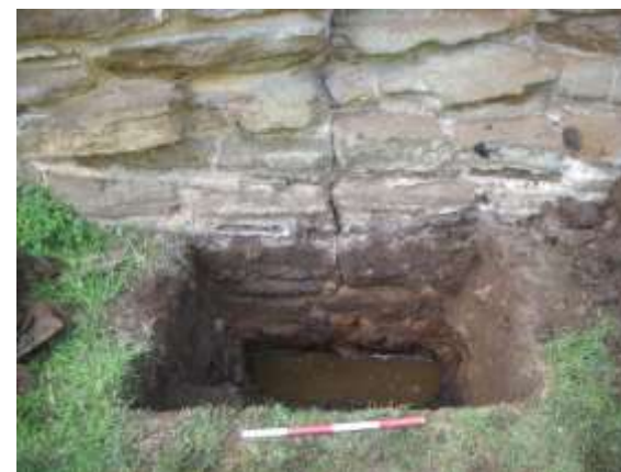
Trench 31: Bathhouse foundations at location of crack 500mm scale
