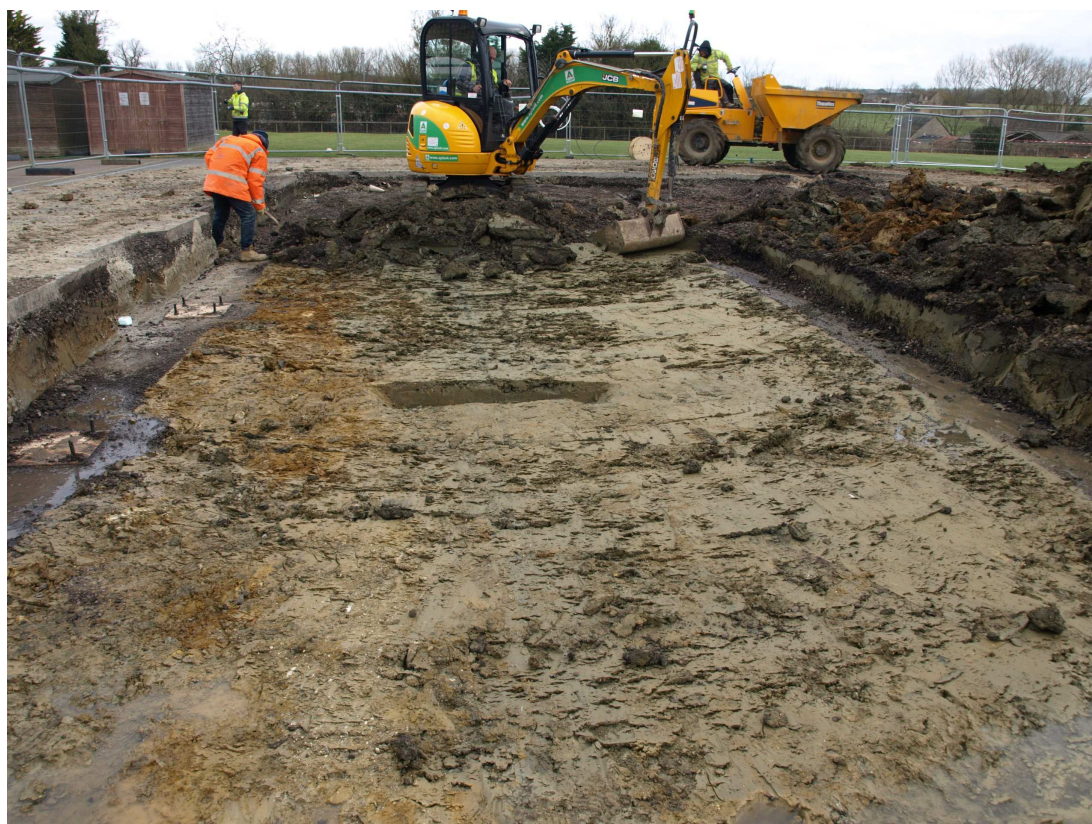
Image 4: General view along furrow [9], looking westwards, during the general ground reduction between the footings
