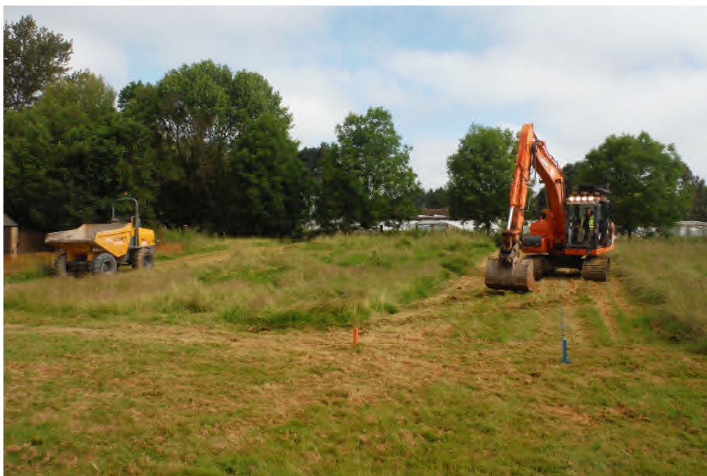
Image 1: General view of the site prior to stripping, looking north with the ground sloping down to the south and west
