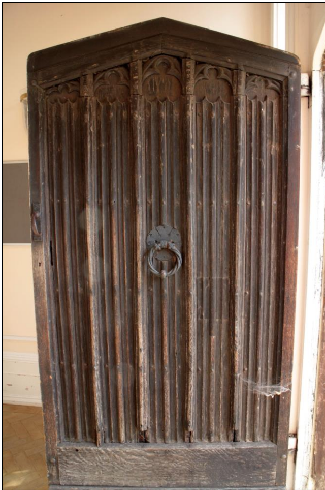
Image 5: Main entrance door External face of door with detail of door knocker below
