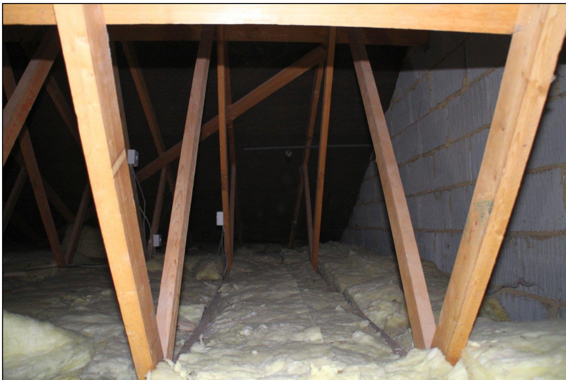
Image 43: Roof space above bathroom and bedrooms 12 and 13 Looking north from hatch in bathroom ceiling showing modern trussed roof and blockwork in gable wall at east end of front range
