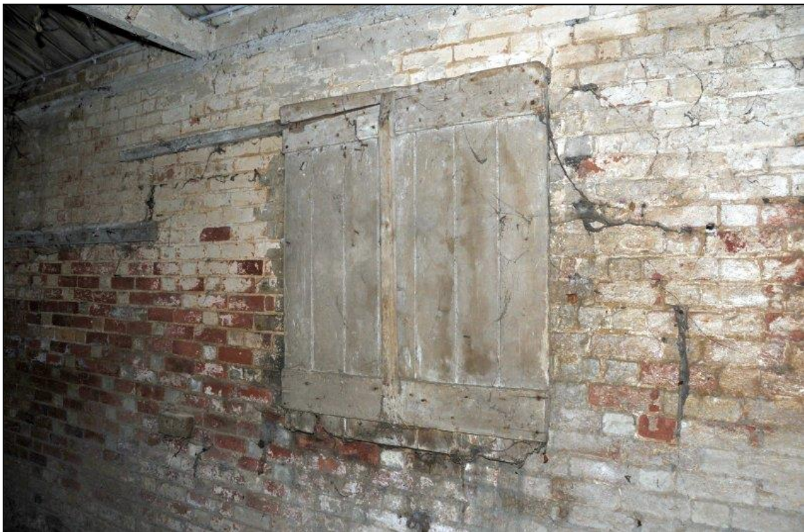
Image 12: South range: C2, detail of shutter on north wall Showing sliding shutter covering window
