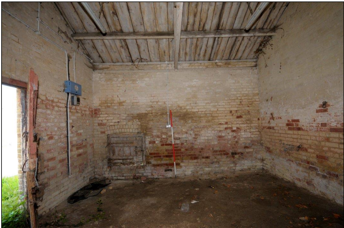
Image 8: South range: C1, looking north Showing low-level opening at end of north wall (Scale 2m)
