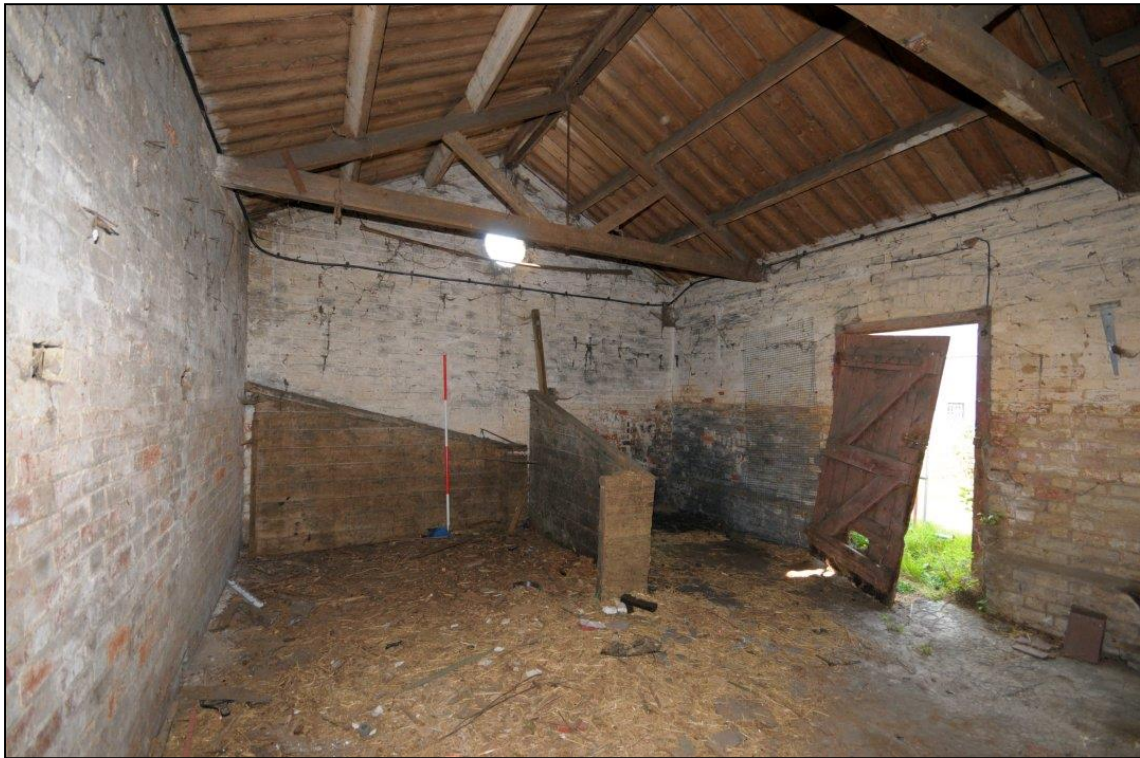
Image 47: West range: C16, looking south-west Showing external door in west wall and stall dividers (Scale 2m)
