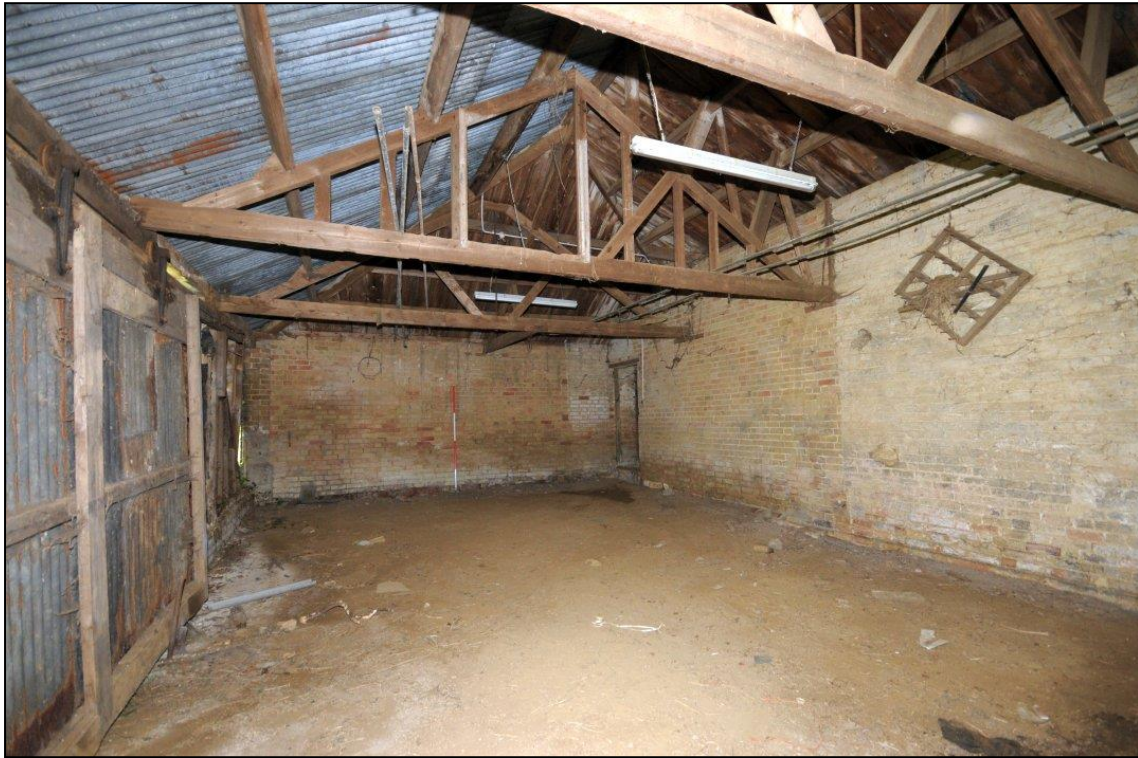
Image 39: North range: C10, looking east Showing rear (south) and end (east) walls (Scale 2m)
