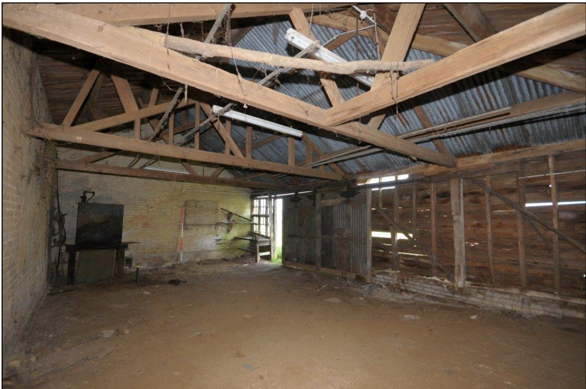
Image 38: North range: C10, looking north-west Showing weatherboard front wall and sliding door (Scale 2m)
