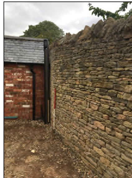
North side of churchyard retaining wall showing ground level difference, 1m scale
