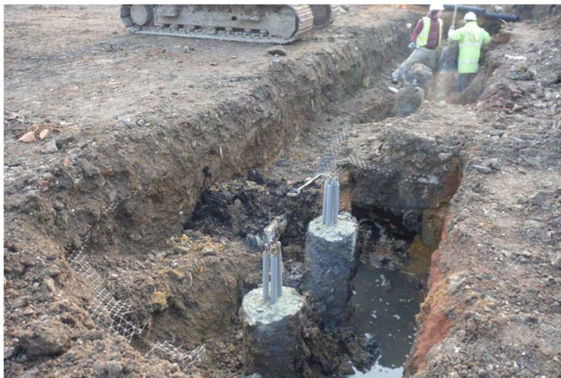
Photograph 3: South wing, south-west edge, heavily truncated by old service trench (black material)
