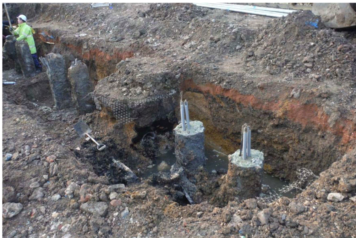
Photograph 4: South wing, south-west edge, heavily truncated by large modern feature and old service trench
