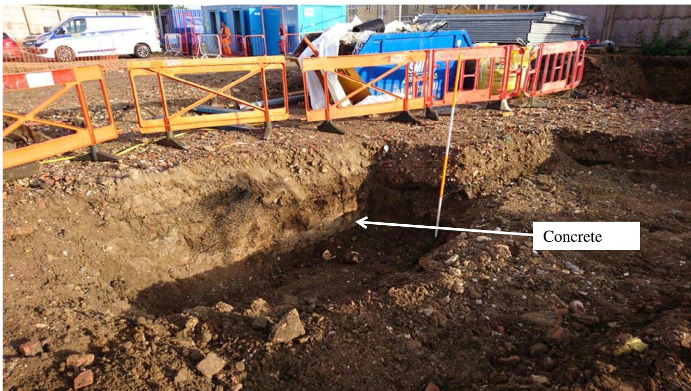
Photograph 16: Test-pit 5 with upper concrete slab in section, top at 28.0m AOD, made ground below
