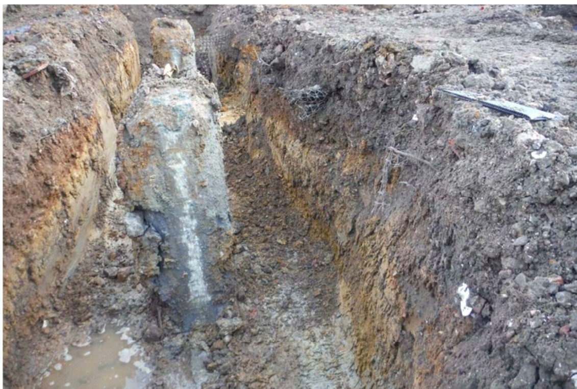
Photograph 1: South wing, beam trench with pile tops – natural sand and gravel surviving
