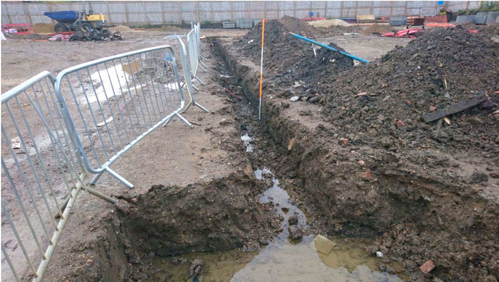
Photograph 11: Service trench on west side of the east wing; entirely excavated into made ground, looking south-east
