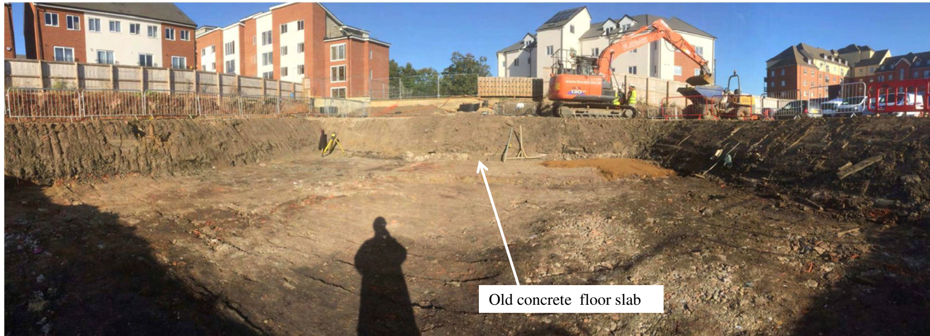
Photograph 12: Attenuation tank, looking north-west; reduced to formation level (c.27.0m AOD), old floor slab visible in section at c.27.1m AOD
