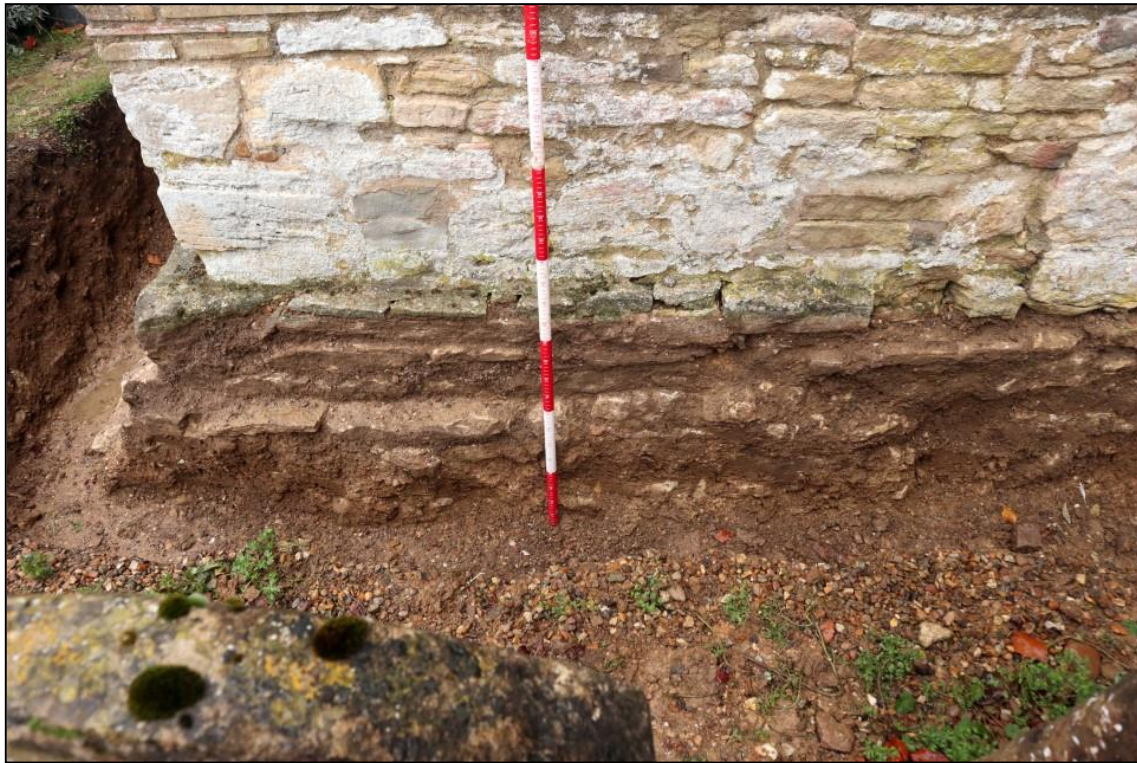
Image 13: Trench 1. East end of south aisle, left end Shows two foundation offsets in rubble masonry (Scale 200mm divisions)
