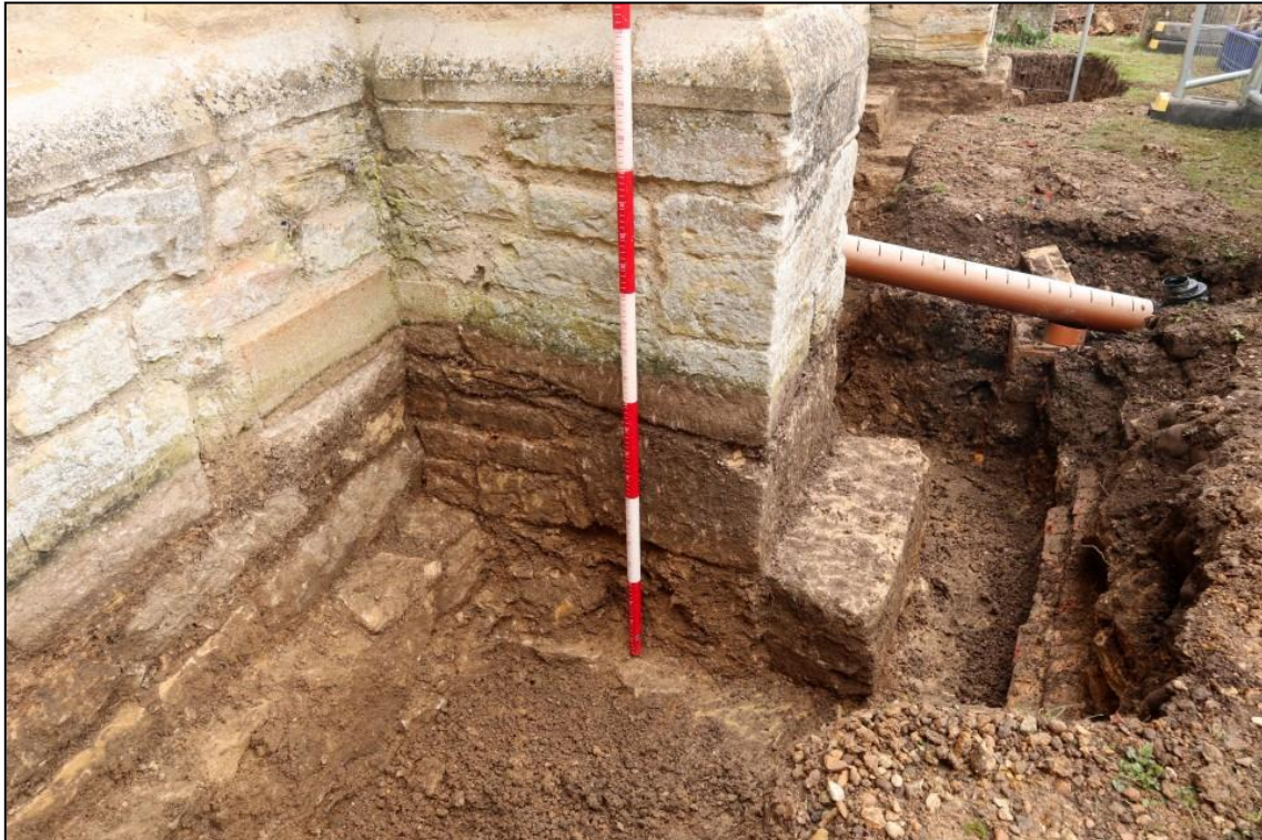
Image 6: Trench 1. South aisle, central buttress, looking north-east Brick vault (104) visible in base of trench at right (Scale 200mm divisions)
