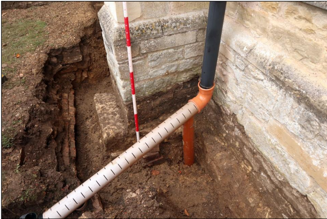
Image 7: Trench 1. South aisle, central buttress, looking north-west Brick vault (104) visible in base of trench at left. (Scale 200mm divisions)
