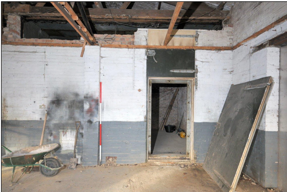
Image 38: Workshop range interior, Workshop 1 Looking north, showing doorway to apple store with the removed door to the right (Scale 2m)
