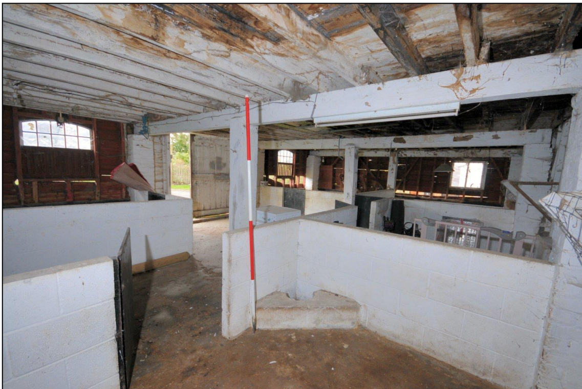
Image 22: Barn interior, ground floor at north end Looking north-west showing blockwork animal stalls (Scale 2m)
