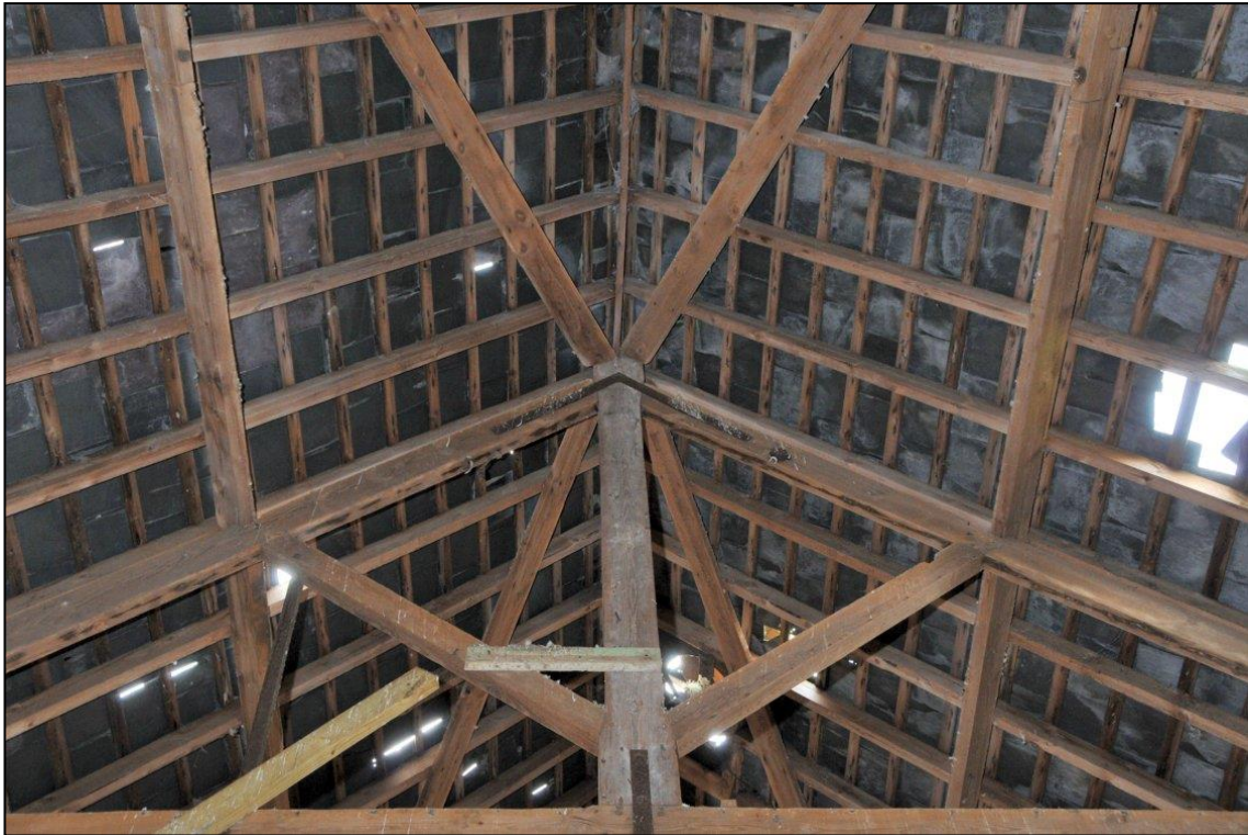
Image 17: Barn interior, detail of roof construction Shows diagonal bracing and one of the trusses.
