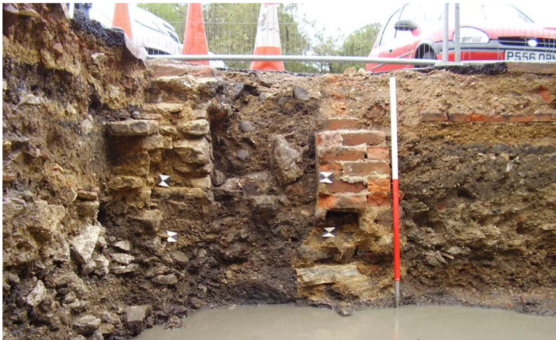
Figure 20: Limestone culvert in the south-east corner of Test Pit 2 (Viewed from the north. Scale 1m)
