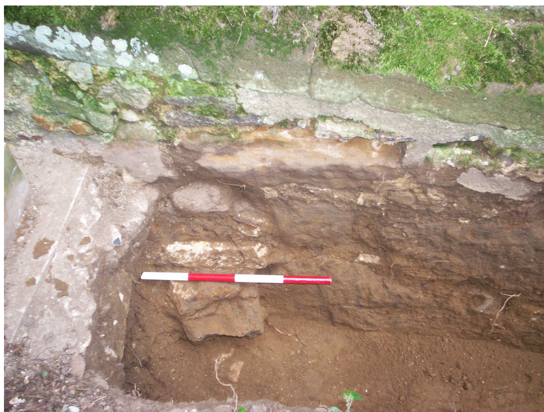
Figure 5: Infilled arched opening (106).
