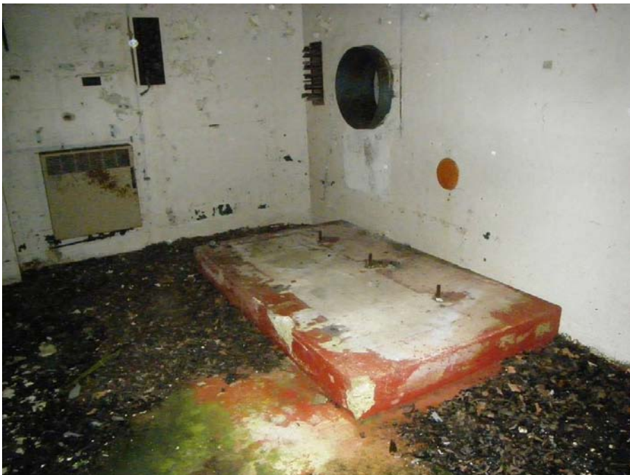
c) SPA8 (pugmill) interior, separate engine room
