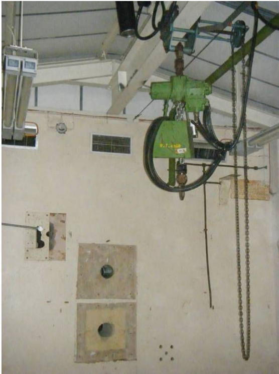
a) SPA48 (pugmill) interior of filling shed hydraulic hoist
