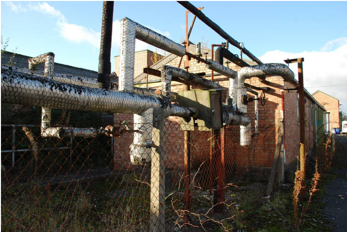
b) Steam heating pipes (SPA1/2 – administration block and canteen)
