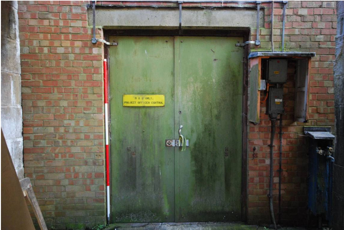
a) SPA21 (rocket motor magazine) metal-clad entry doors, external electrics, stand pipe, lightning protection
