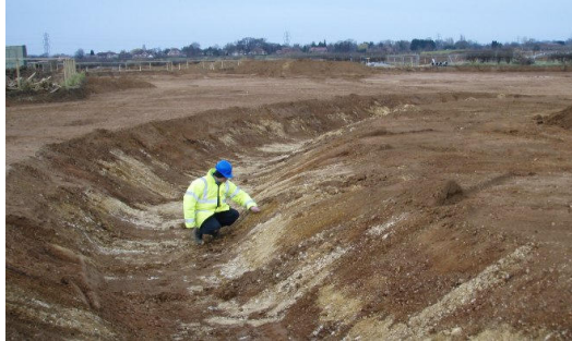
After the completion of hand excavation, the fills of all Bronze Age ring ditches have been machined out
