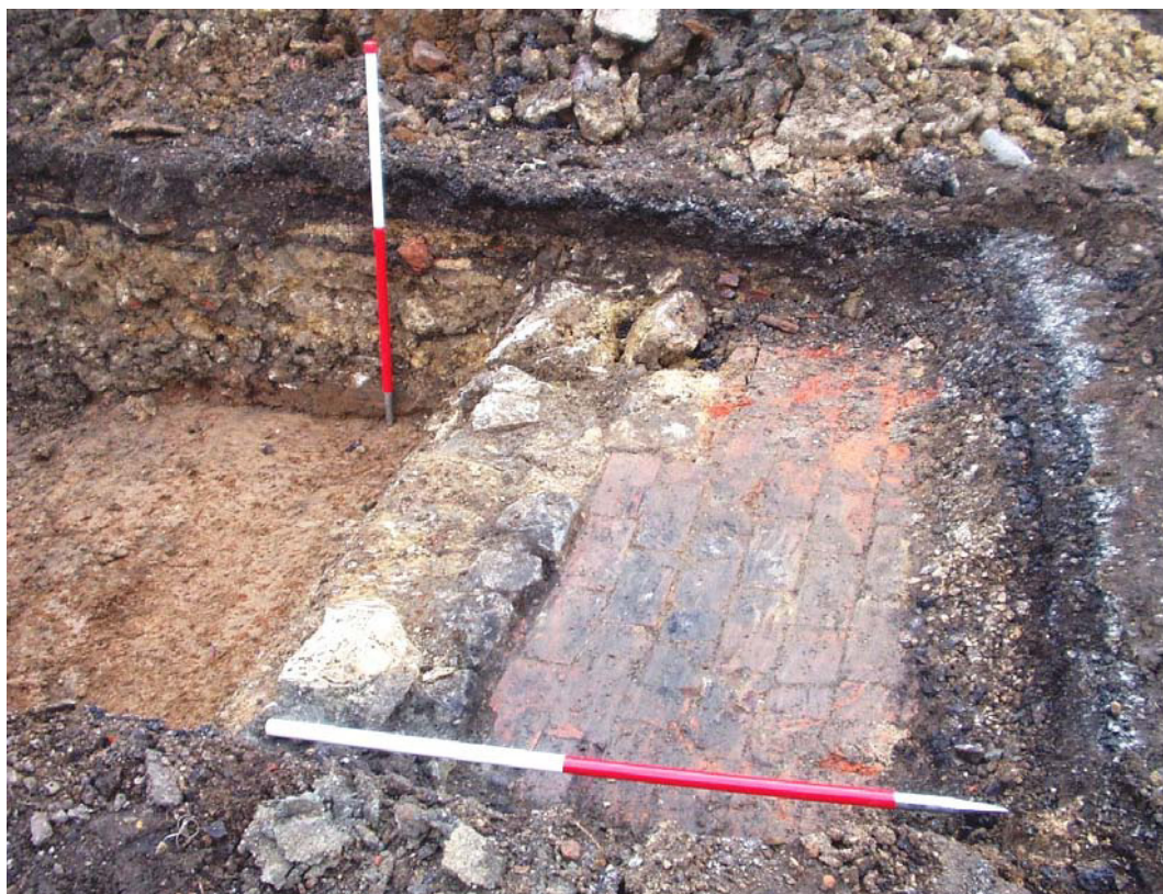
Photograph 7 Western end of Trench 2 showing rear wall of cottage (219) and associated internal tiled surface (220) with construction deposits to left. Discoloration in base of trench is upper surviving fills of the recut substantial ditch. Scales 1m in 0.5m divisions
