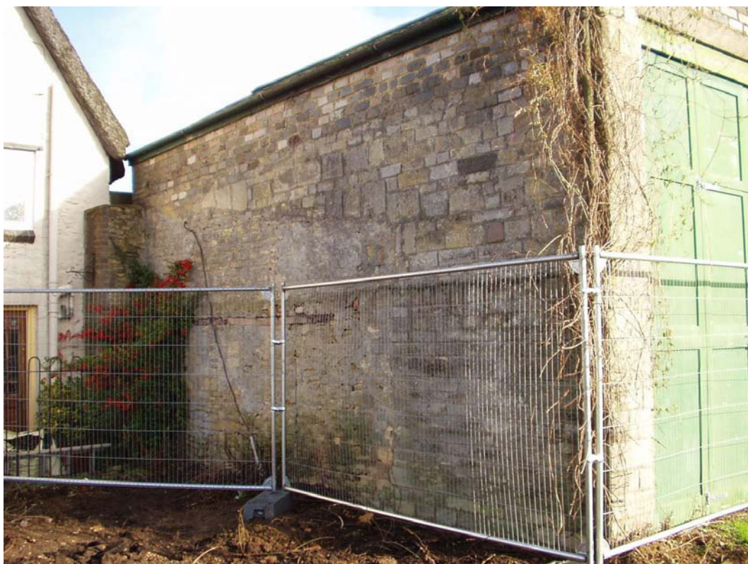
Photograph 2 Western elevation of standing structure showing earlier limestone building incorporated into shed.
