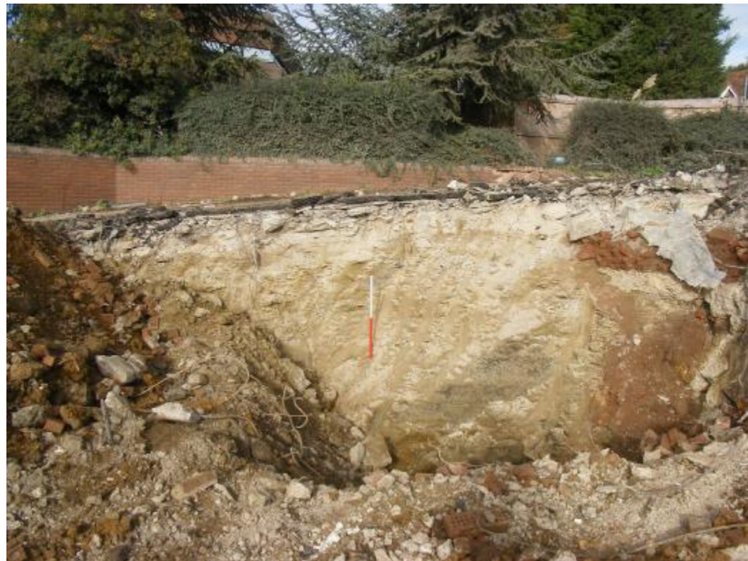
Plate 3: Zone 2/4, preserved limestone deposits after removal of retaining wall adjacent to car park ramp facing north-west. 1m scale
