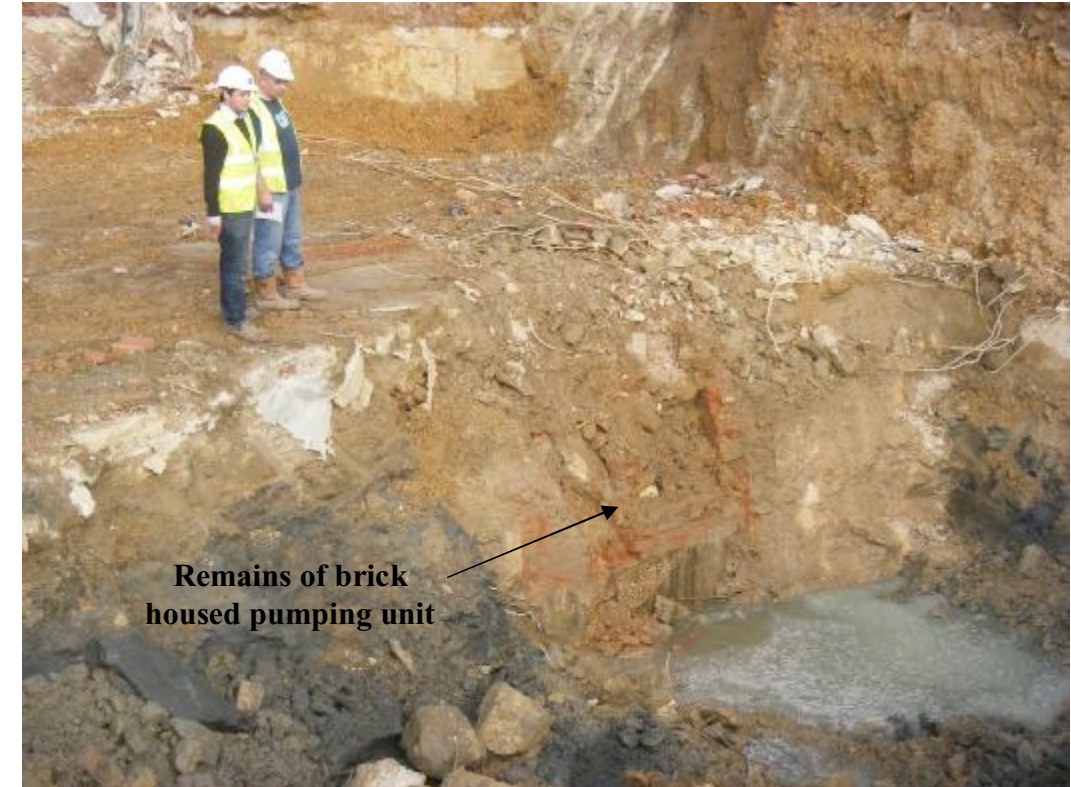
Plate 6: Zones 2-3 facing north-east showing depth of impact of previous building immediately following removal of foundation slabs. 1m scale
