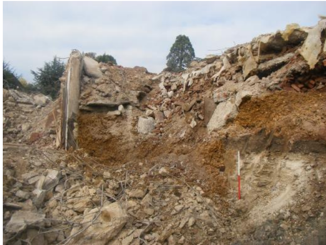
Plate 1: Zones 2-3, partially removed retaining wall facing north showing preserved subsoil and limestone deposits. 1m scale
