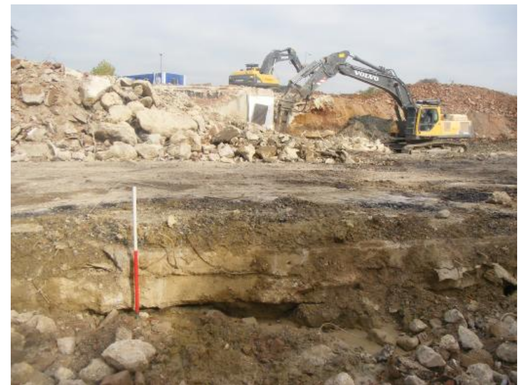
Plate 8: Zone 2 facing north-east showing depth of concrete slabs overlying clay geology. 1m scale
