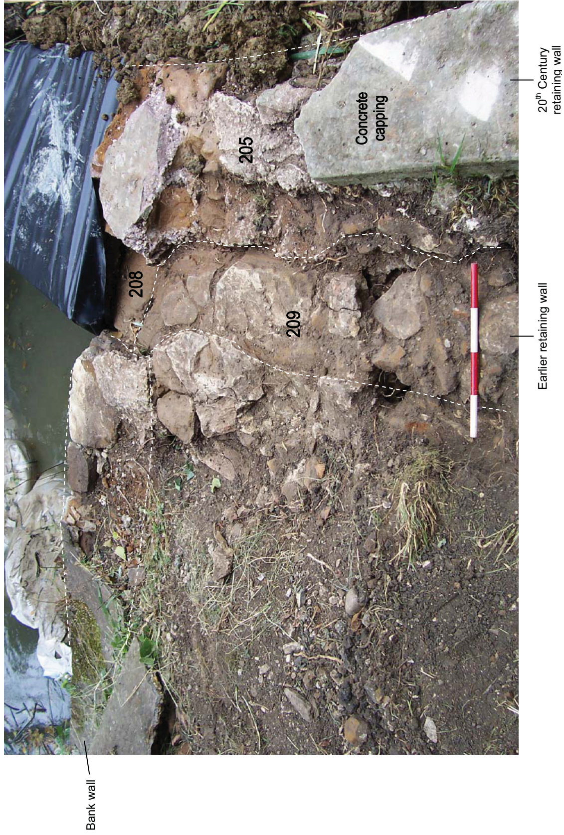
Figure 5: Junction of eastern bank wall, weir wall (208), 20 th century retaining wall (205) and earlier retaining wall (209). Scale 40cm
