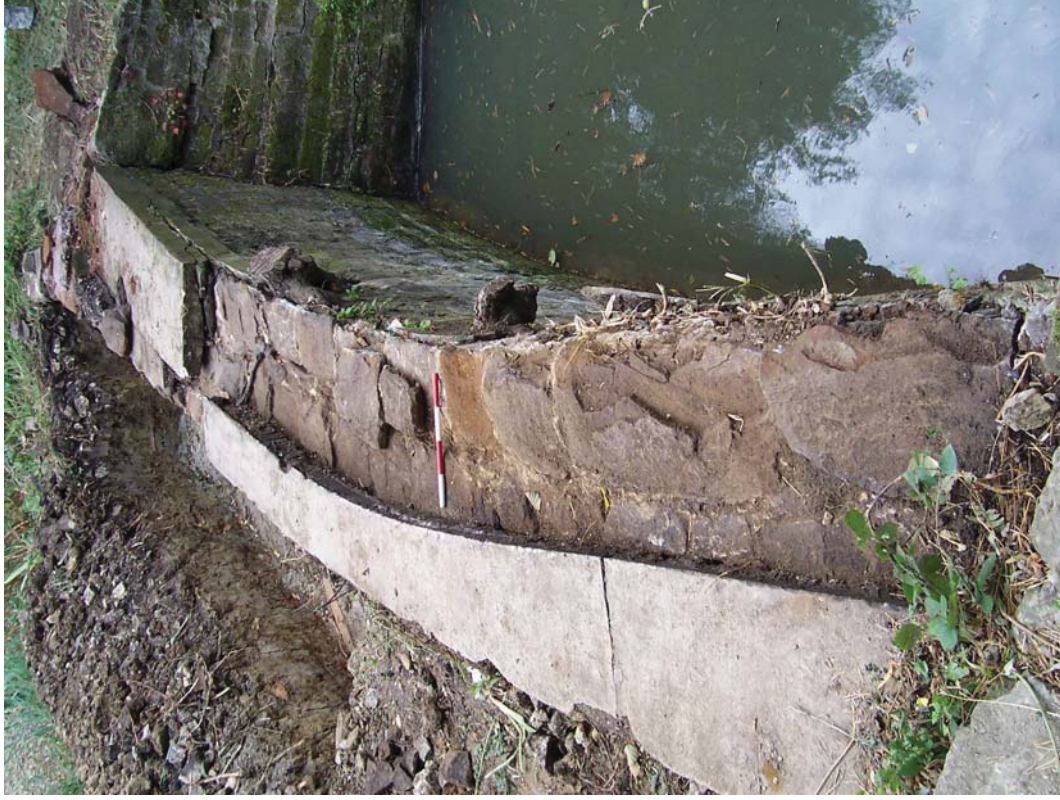
Top of weir wall (208) after removal of concrete capping. Looking east. Scale 40cm
